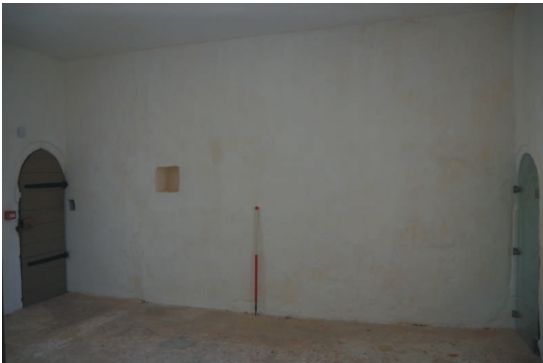
Plate 5: South wall showing scar, looking south-southeast (1m scale)
