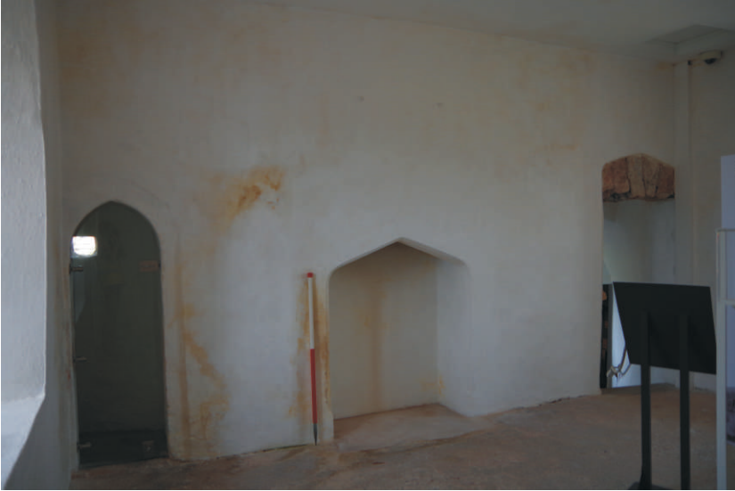
Plate 1: North wall showing fireplace and wall scar adjacent to door, looking north-northeast (1m scale)
