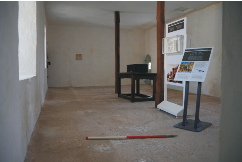
Plate 2: General view showing scars on the floor and south wall, looking southwest (1m scale)
