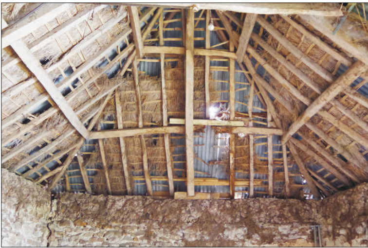
Plate 5: General view of north end of the roof, showing repairs, looking north
