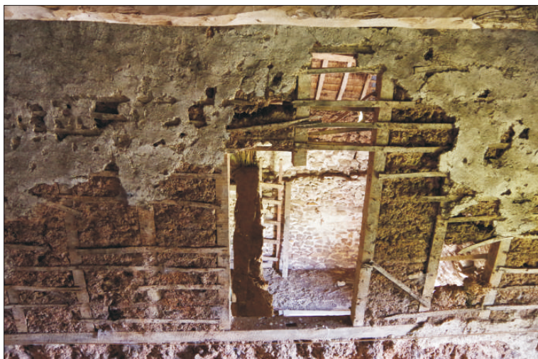
Plate 3: Central part of the partition wall showing the removed stud and socket in the beam below, looking south
