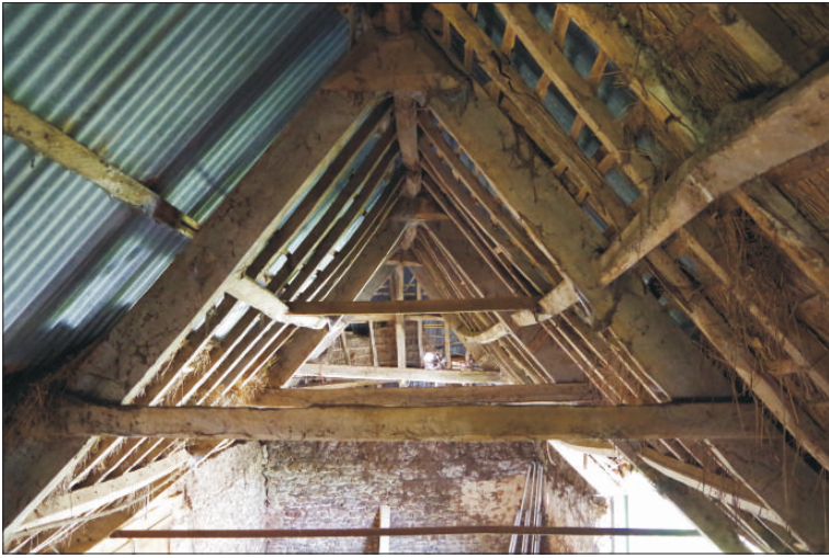
Plate 4: General view of roof trusses, with truss 4 in the foreground, looking north
