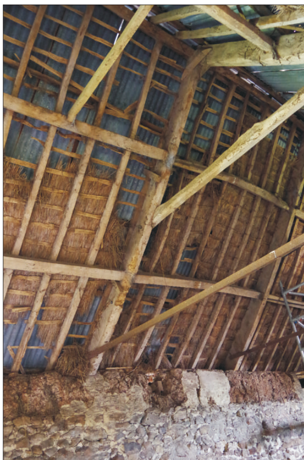
Plate 8: General view of roof showing trusses 3 and 4 and areas of thatch, looking southwest
