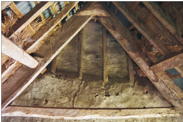
Plate 2: Top part of the partition wall and the upper part of roof truss 5, looking south
