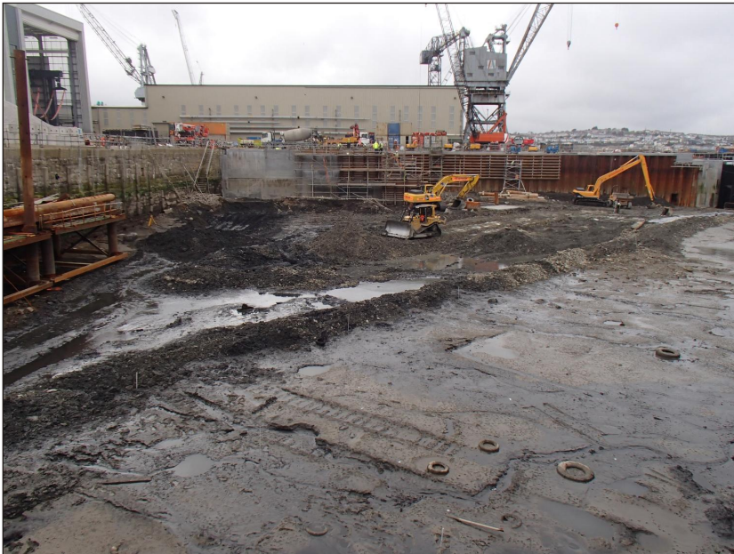
Plate 2: The drained wet basin during removal of foreshore silts, viewed from east
