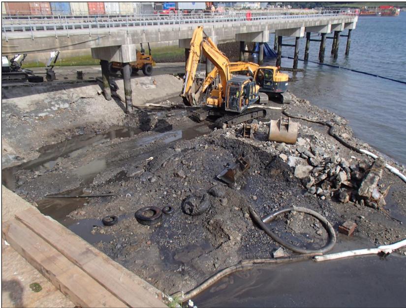
Plate 1: General shot of initial removal of foreshore silts, viewed from the southeast
