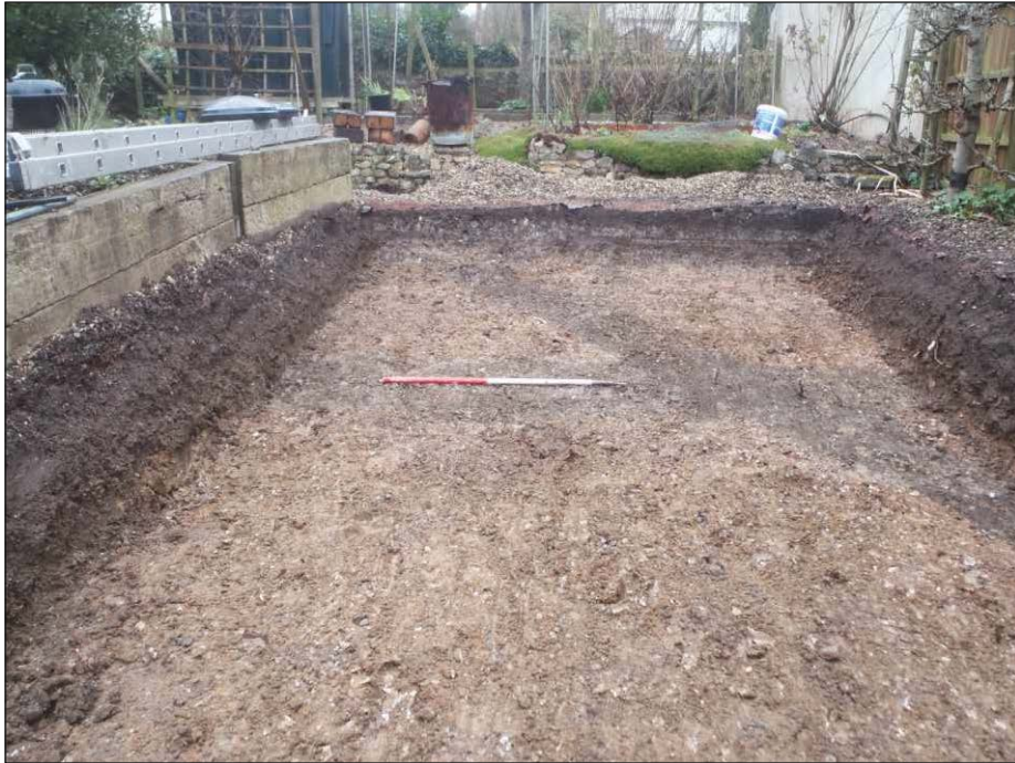
Plate 1: Showing area for new garage and water filtration system. Looking northwest towards ditch F106 (scale 1m)
