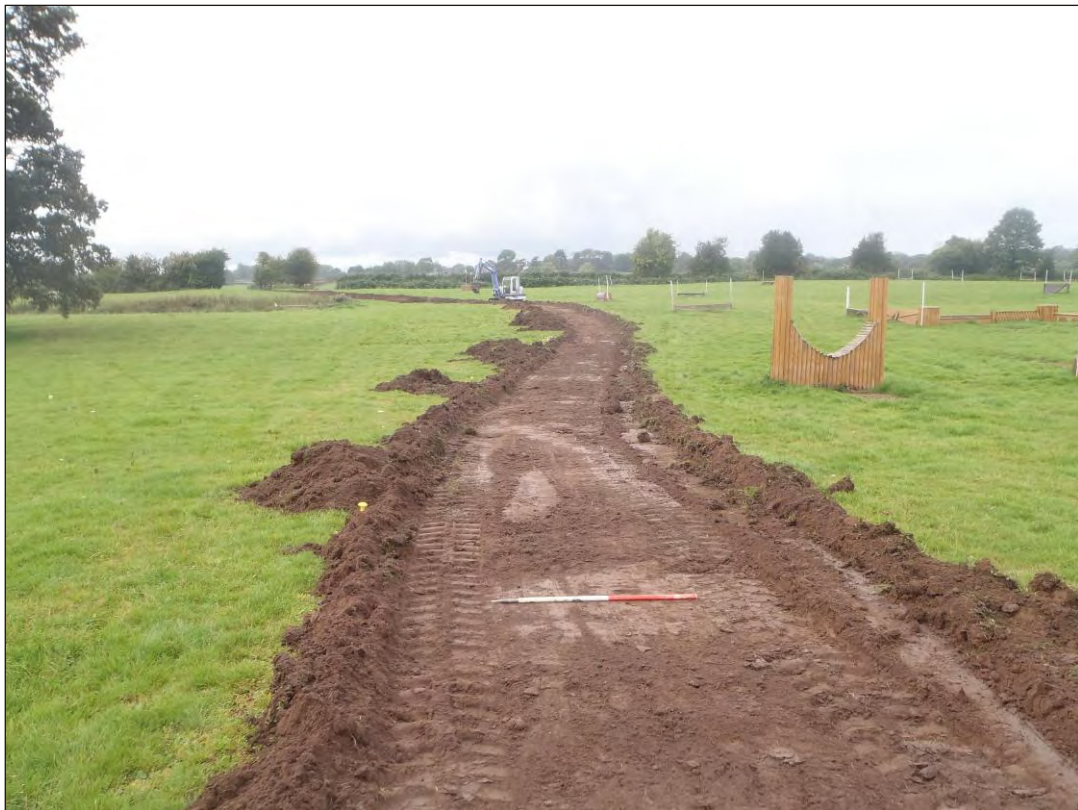
Plate 2: General view of new access road during topsoil stripping, looking to the west (1m scale)
