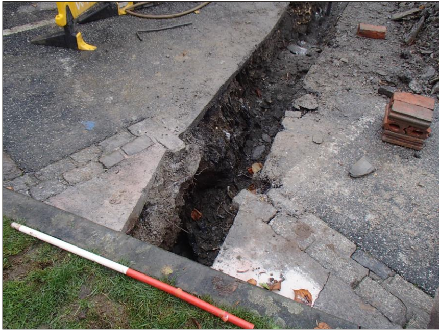
Plate 1: Trench 1, general view showing the high level of natural bedrock, looking southeast. 1m scale
