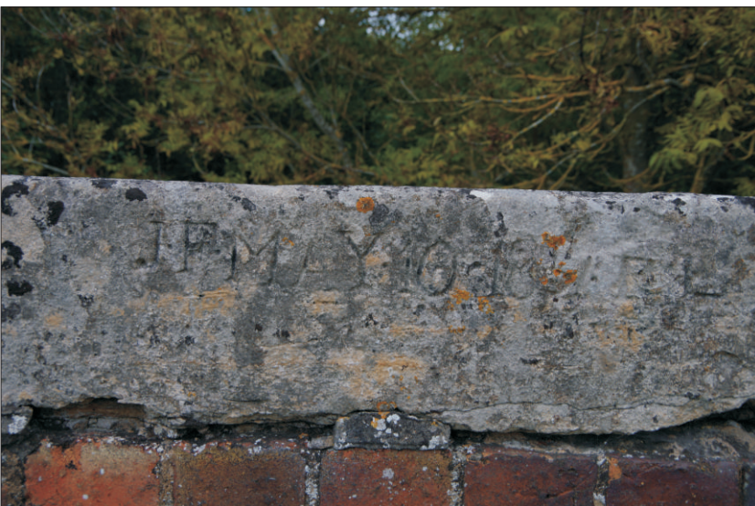
Plate 14: View of inscription which appears to read 'IF MAY 10.18 IF', seen on a capping block on the north side of the bridge
