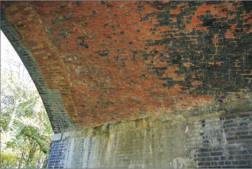
Plate 12: View of brick repairs to the roof of the central arch, looking east
