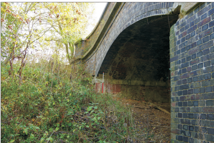
Plate 6: View of one end of the bridge emphasised by projecting forward by two courses of brickwork, looking southeast (1m scale)
