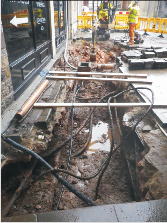
Plate 1: Castle Bow trench, Castle Walk, with work in progress, view from the north
