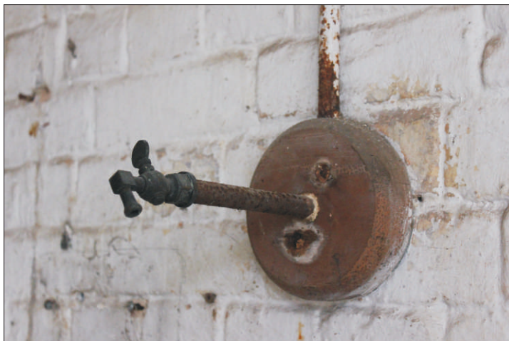
Plate 8: Gas fitting in south garage in The Morgue, looking northwest
