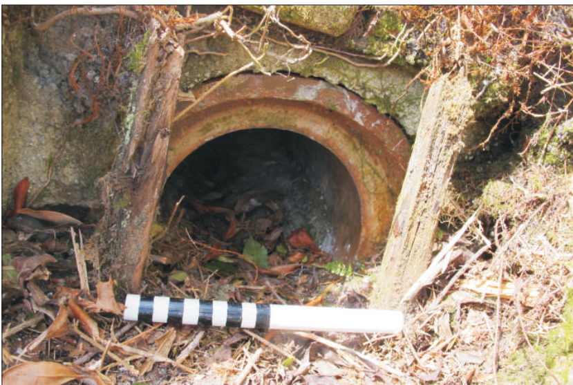
Plate 12: Inflow (RSP2.1) earthenware pipe and wood posts for control hatch, from southeast (0.20m scale)
