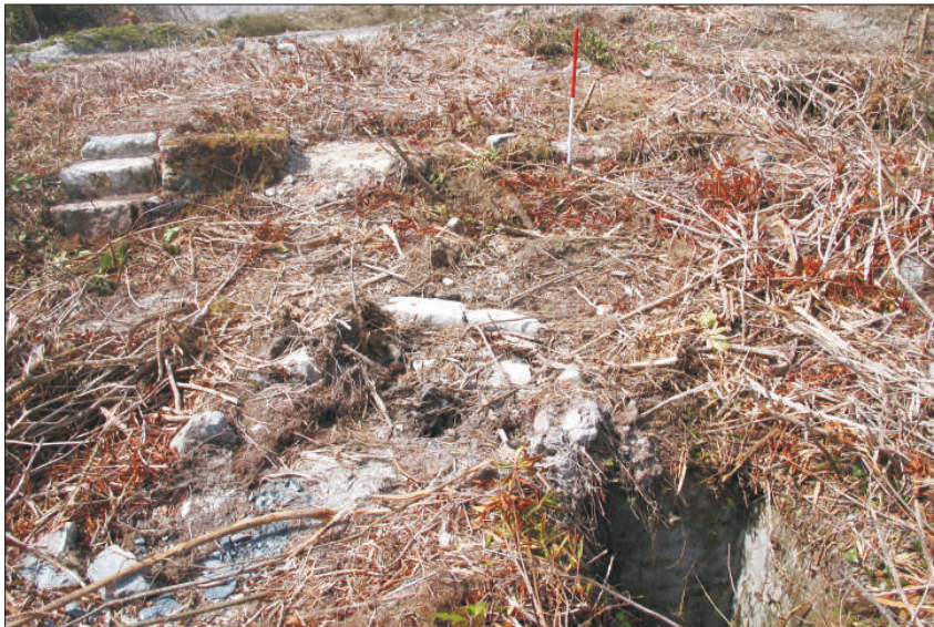
Plate 21: Demolished area, strewn with debris, from east. The cement-lined pit (DA.2) is in the foreground (1m scale)
