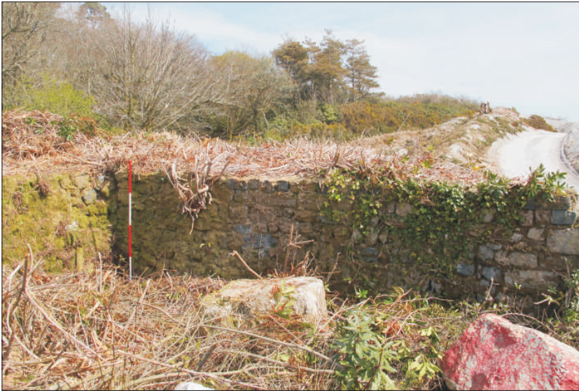
Plate 14: Settling Tank interior east wall, with corner on left and dressed stones to the right, from west-southwest (2m scale)
