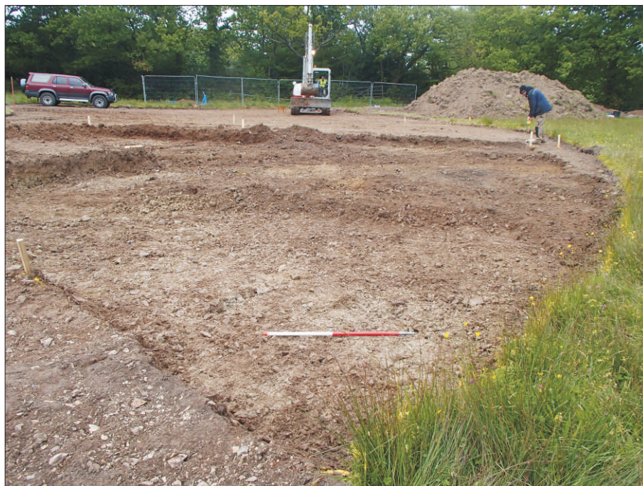
Plate 2: Working view of stripped area for county house. Looking southeast (scale 1m)
