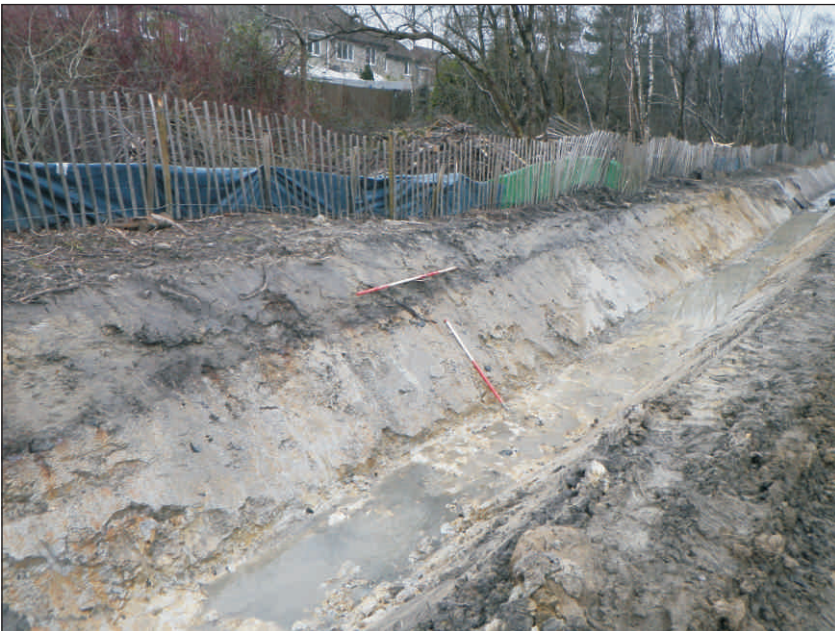
Plate 2: General view of new drainage trench, looking to east. Scales 2m and 1m
