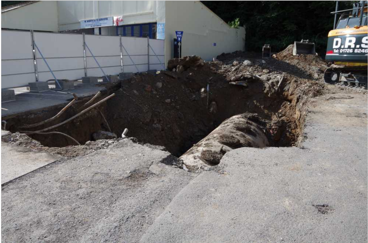
Plate 1: Glen Lyn Car Park (Area 1), general view during initial removal of fuel tanks
