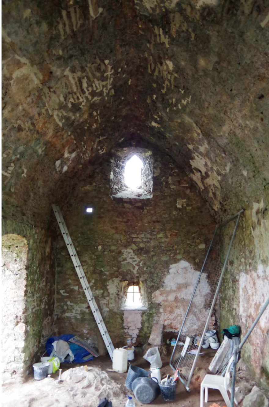
Fig. 14: St Michael's Chapel, Torre interior, during conservation works, showing vaulted roof and west end
