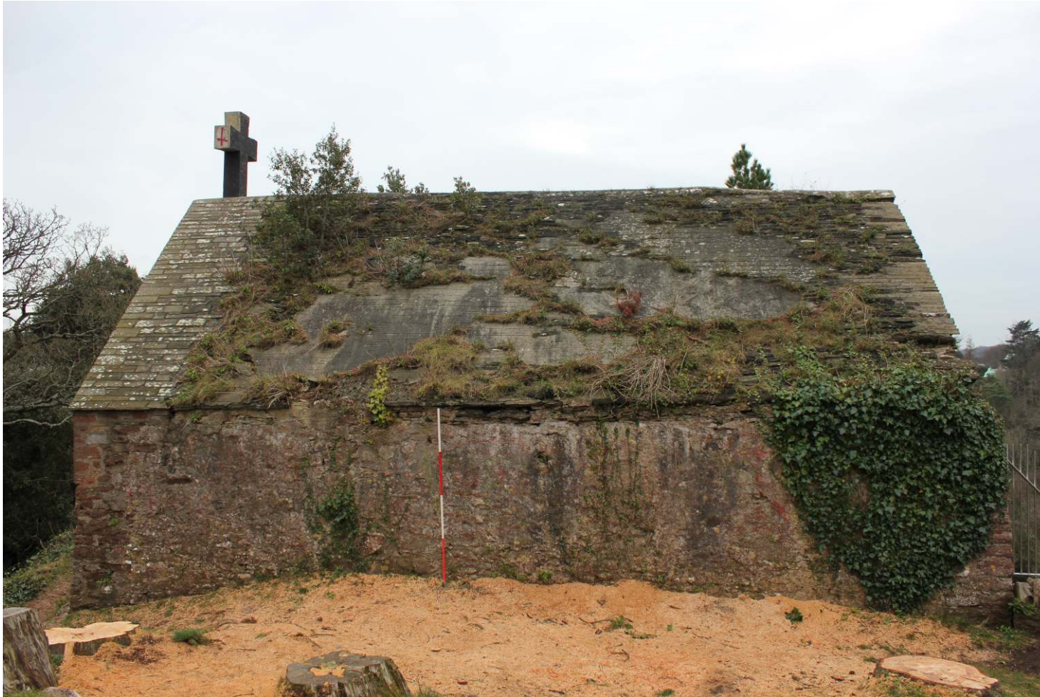
Fig. 3: St Michael's Chapel, Torre prior to conservation works. Viewed from the north (2m scale)
