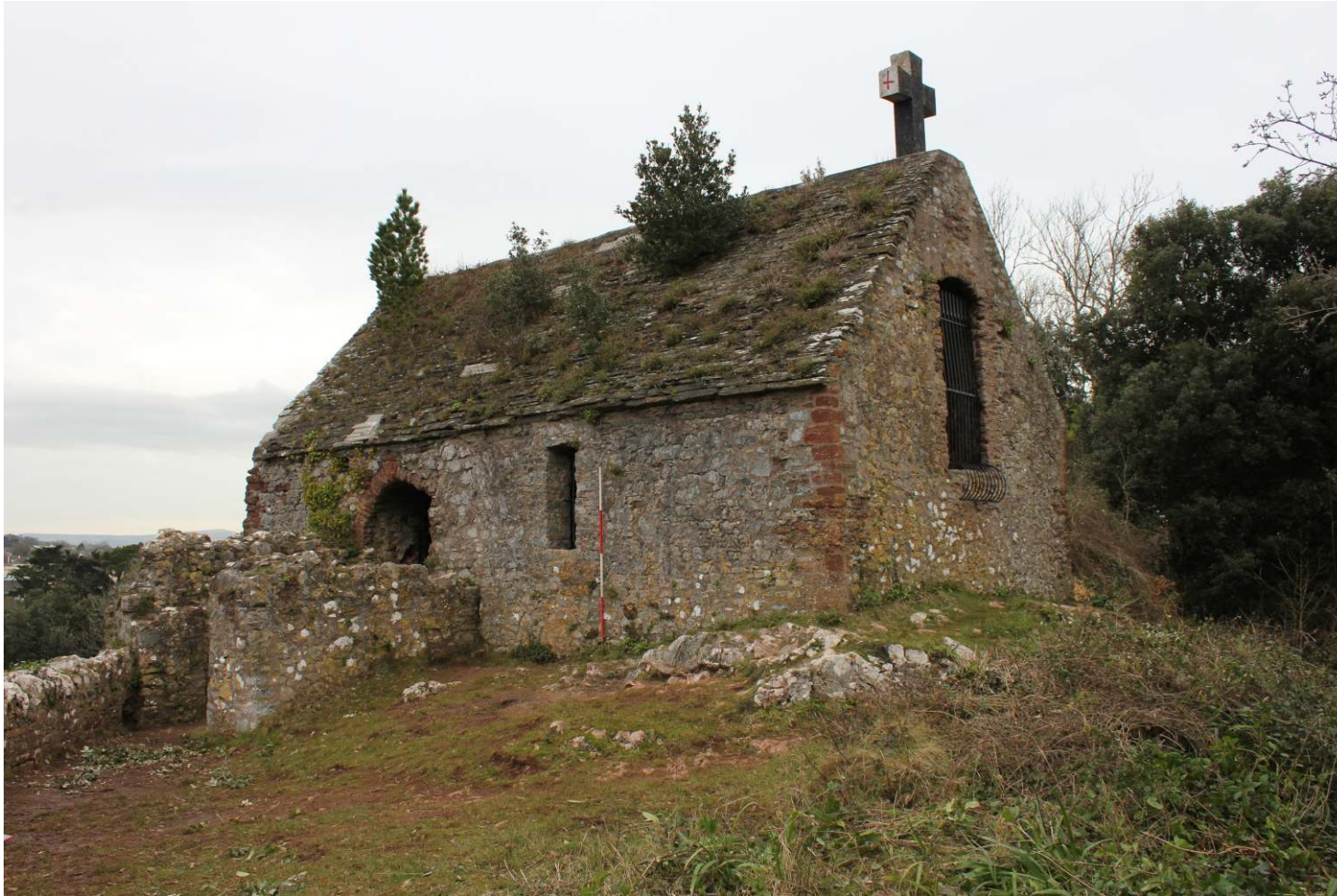
Fig. 2: St Michael's Chapel, Torre prior to conservation works. Viewed from the south-east (2m scale)
