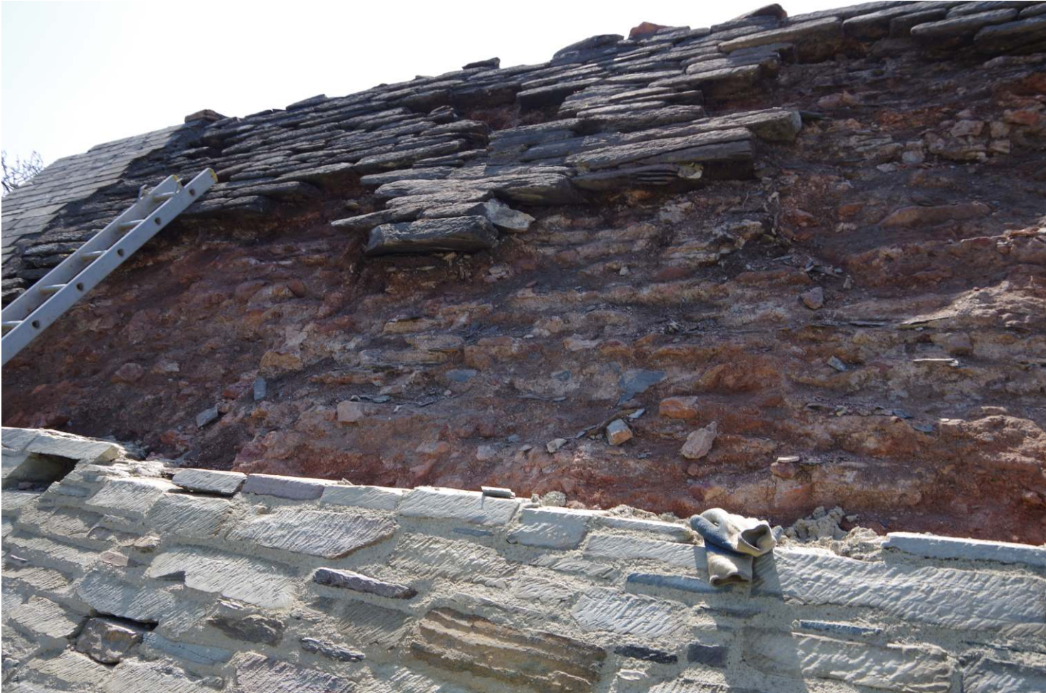
Fig. 13: St Michael's Chapel, Torre northern pitch during conservation works, showing vaulted roof core material
