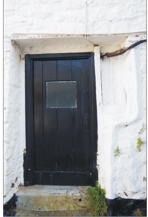
Plate 6: Door and earlier window in the southwest elevation of the rear range, looking northeast
