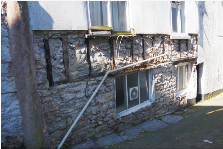
Plate 3: Ground floor of the northeast elevation of the central range showing the timber framing, looking northwest
