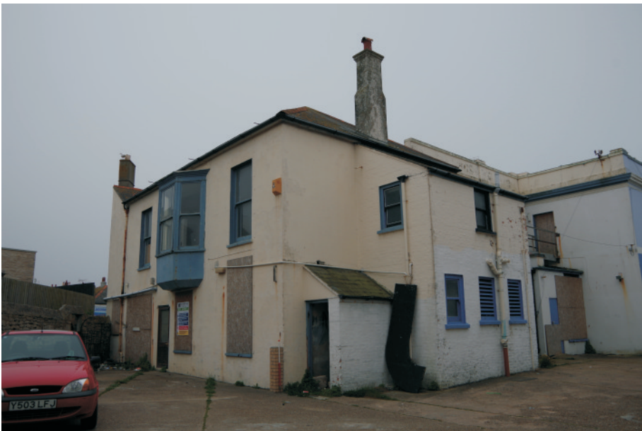
Plate 5: The east elevation of the east block and the north and east elevations of the brick extensions, viewed from the northeast. 1m scale.
