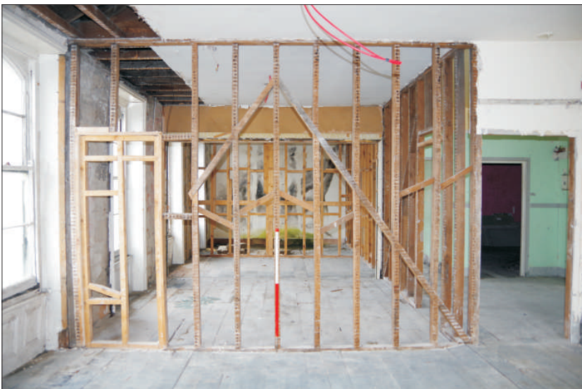
Plate 25: General view of bathrooms 3 and 4 (stud wall between them removed) with bedroom 11 at the back taken from the office, looking north (1m scale)
