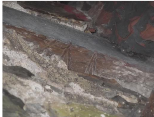
Unidentified markings under tiles
