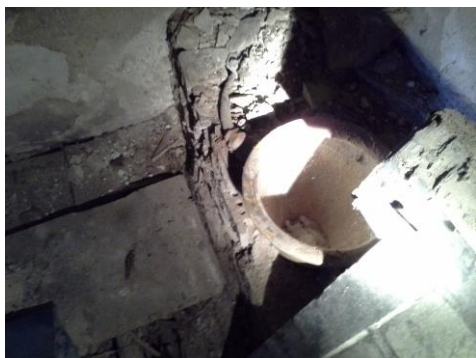
Cell sanitary fitting
