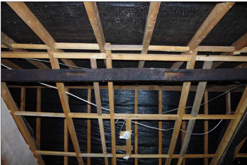
Plate 16: Detailed view of empty sockets in the purlin with wooden pegs for supporting a wind brace, looking north
