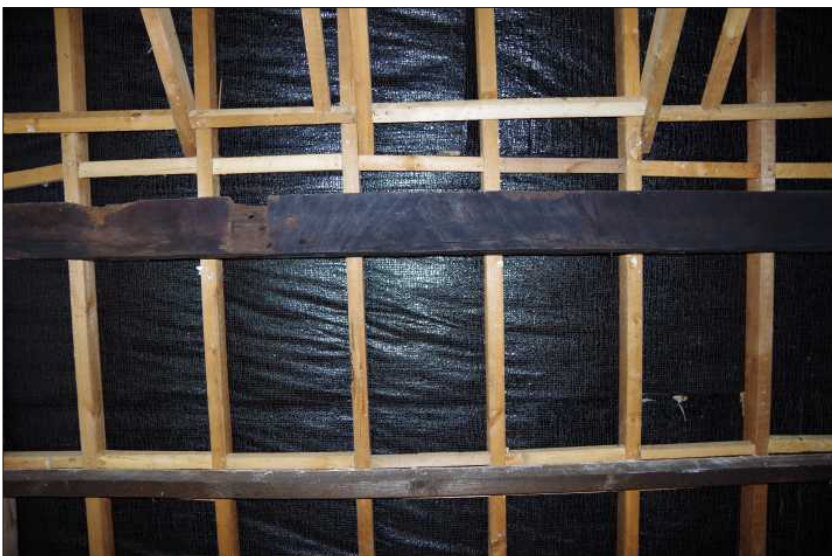
Plate 17: Detailed view of empty peg holes in the purlin for supporting a wind brace, looking south
