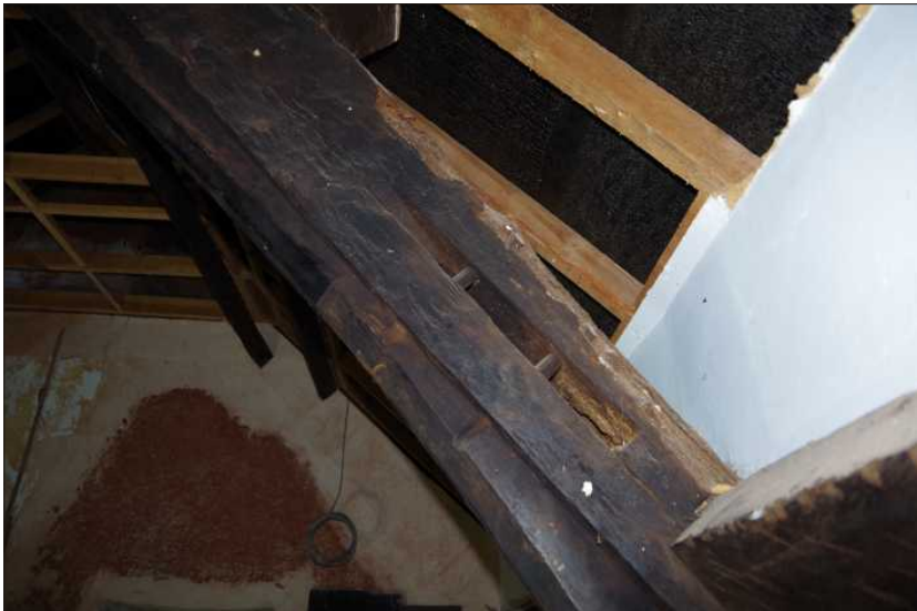
Plate 15: Detailed view of empty socket in the truss with wooden pegs for supporting a wind brace, looking west
