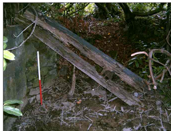
Plate 3: Mount Foundry Leat, remains of sluice structure at junction with Town Leat, view from the south (scale 1m)
