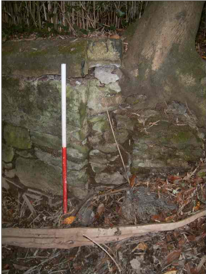
Plate 4: Mount Foundry Leat, slot in leat wall for collapsed sluice structure at junction with Town Leat, view from the east (scale 1m)
