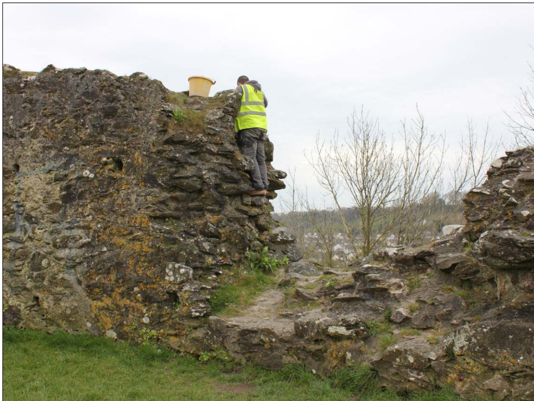
Plate 4: General location of stones 2 and 3 viewed from within the keep during replacement of stone 2, looking east
