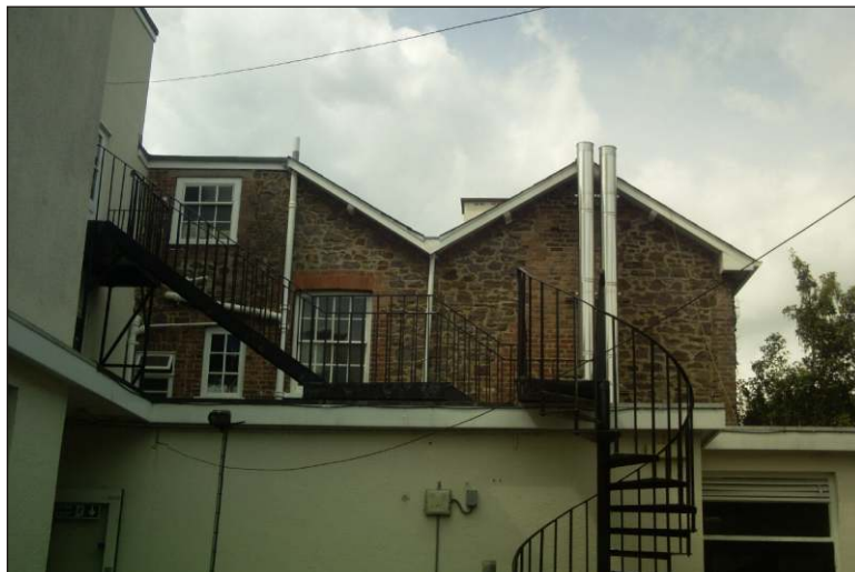
Plate 3: The east elevation showing the first-floor masonry above late 20th-century extensions, looking west
