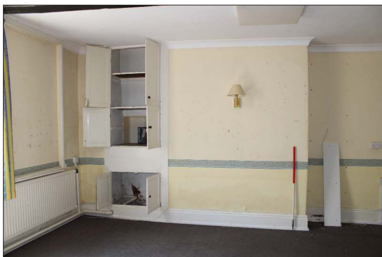
Plate 9: Room 4 showing rear of chimney stack and adjacent cupboard, looking west. (1m scale)
