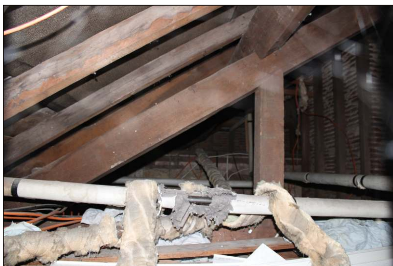
Plate 21: The rear central roof viewed from a hatch in WC4, looking south
