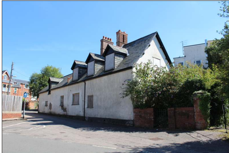
Plate 22: The north elevation of the outbuilding, also showing the gates into the property, looking southeast
