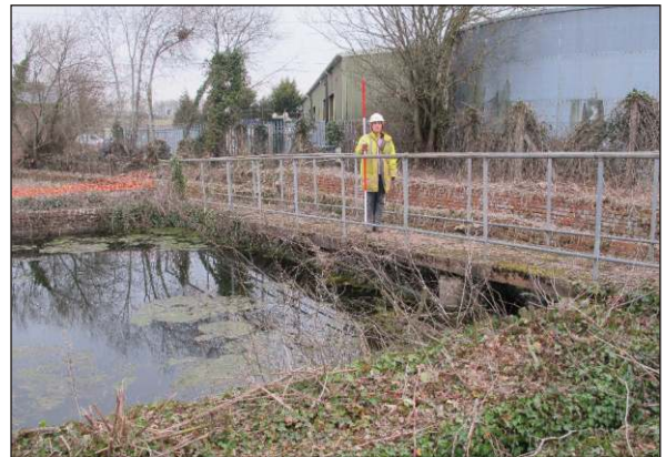
Plate 64: Concrete footbridge F10 at northeast end of main settling tank T1, with channel C3 in foreground and channels C1b and C2 behind, from south. (2m scale)
