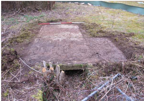
Plate 63: Stone slab bridge F6 over channel C1a between buildings GR1 and L1, from east. Drilled holes are seen in the main slab. (2m scale)
