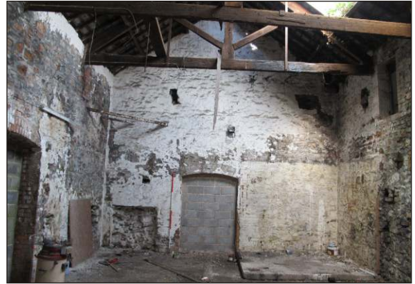
Plate 16: Building GR2 interior of Room B, showing blocked doorway in northwest wall, iron corner bars and roof timbers, from southeast. (2m scale)
