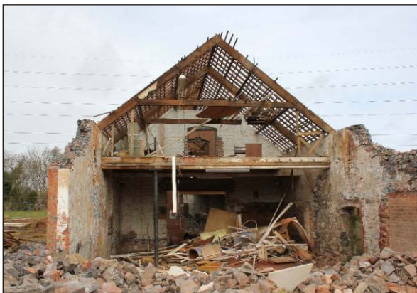
Plate 11: Building GR1 partly demolished section showing Room A with roof timbers and iron pillar supporting upper floor, from southeast
