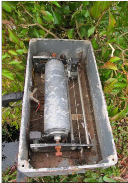
Plate 61: Chart flow recorder box F1 interior, with chart drum and pen assembly, from southeast
