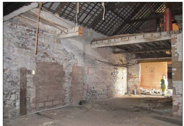
Plate 12: Building GR1 interior of Room B showing northeast wall, blocked doorways, sawn off upper floor timber, and opening to passage, from west. (2m scale)
