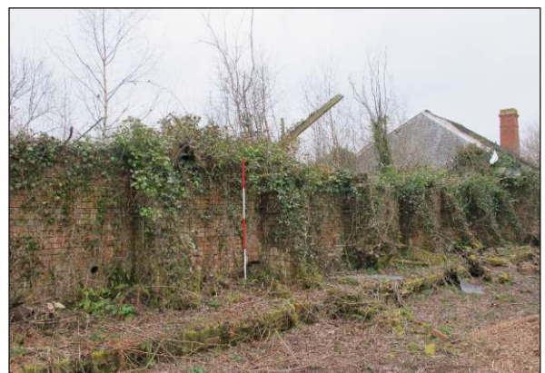
Plate 48: Buttressed Filter Tank (BFT) exterior of northwest brick wall, with filter bed B1 in foreground, from north. (2m scale)
