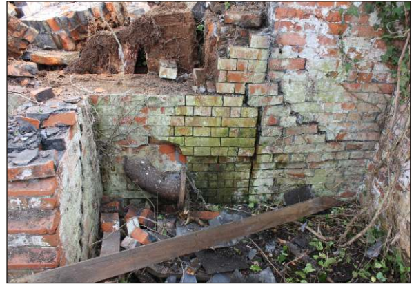
Plate 52: Buttressed Filter Tank (BFT) exterior of southwest wall, with iron pipe from chamber 8 into northeast wing of Building L1, from west
