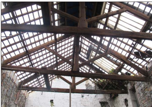
Plate 17: Building GR2 interior of Room B, showing roof timbers with slates removed, from southeast
