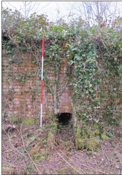
Plate 49: Buttressed Filter Tank (BFT) exterior of northwest wall and sluice outlet from chamber 3, from northwest. (2m scale)
