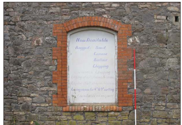
Plate 6: Building GR1, southwest elevation, detail showing the quality of brickwork around the third window, from southwest. (2m scale)
