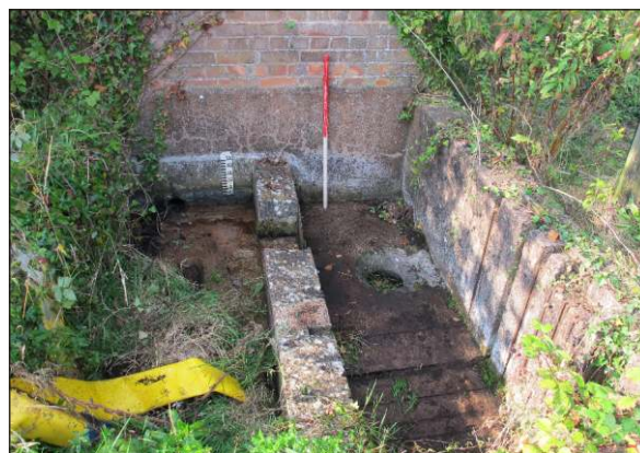
Plate 65: Small gauge tank F11, outside main pump house PH1 partly cleared, from northeast. (1m scale)
