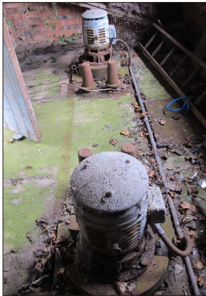
Plate 39: South pump house PH2 interior with two pumps, from northwest
