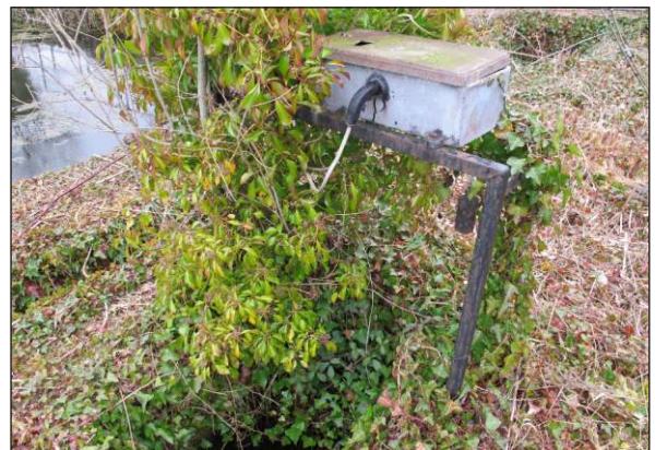
Plate 60: Chart flow recorder box F1 related to channel C3 on southeast side of settling tank T1, from south-southwest
