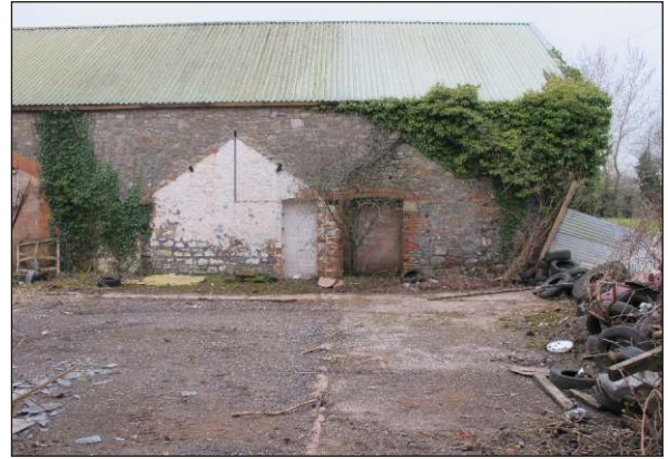
Plate 8: Building GR1, northeast wall, with blocked doors and trace of attached buildings GR7 (left) and GR4, including foundation line, from northeast
