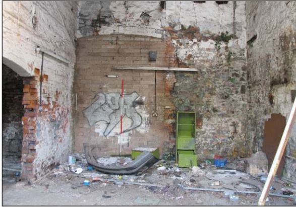
Plate 15: Building GR2 interior of Room A showing blocked arch in northeast wall, from southwest. (2m scale)
