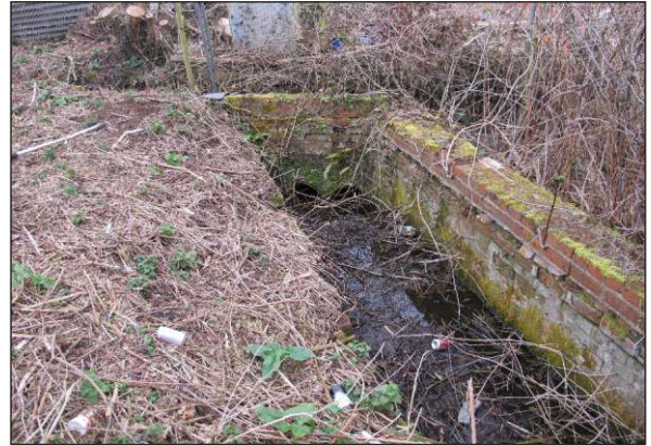
Plate 58: Channel C2 culvert pipes beneath overgrown corner of C1a and C1, from southeast
