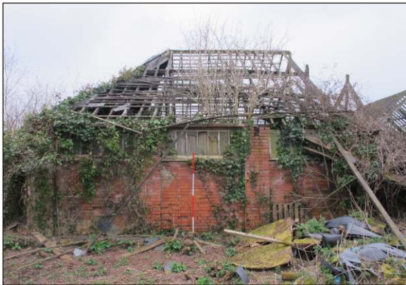
Plate 27: Building L1, northeast wing exterior with raking stretcher bond brickwork and windows, from northwest. (2m scale)
