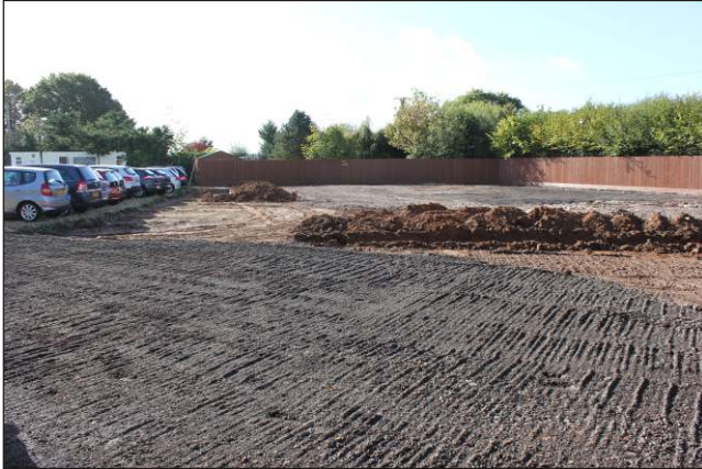
Fig. 1: General view of the site looking south. The depth of topsoil removal is visible to the rear of the cars.
