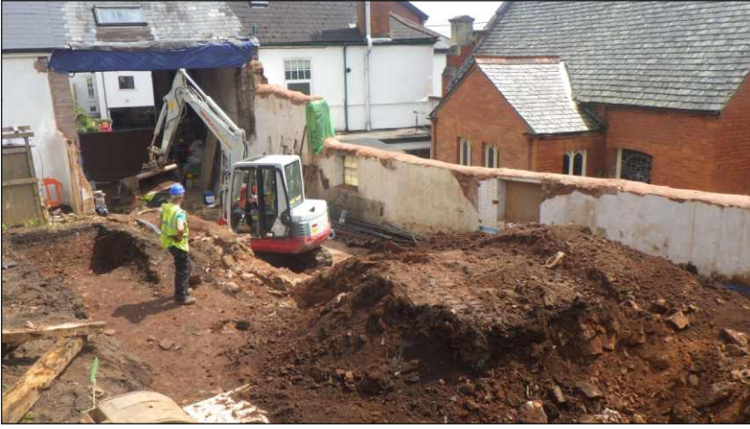
Plate 13: General working view during groundworks following demolition of workshop range. View to southeast
