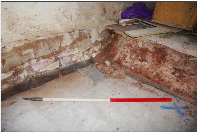
Plate 8: Showing reduced floor level and wall scar. View to south (scale 1m)
