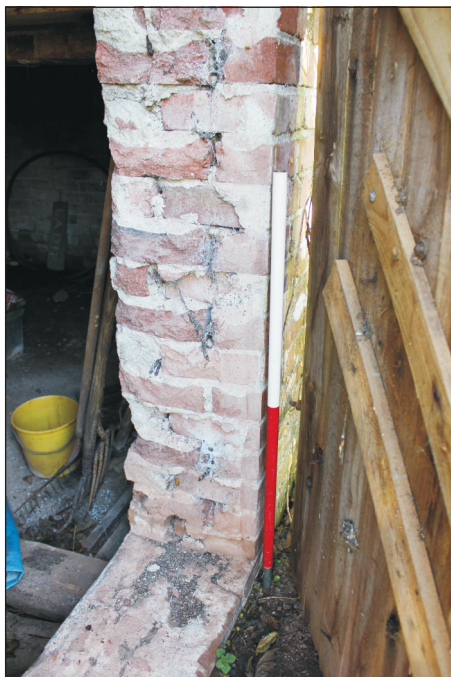
Plate 11: The modern rear opening to shelter showing the reinforced brickwork, looking east-northeast. (1m scale)
