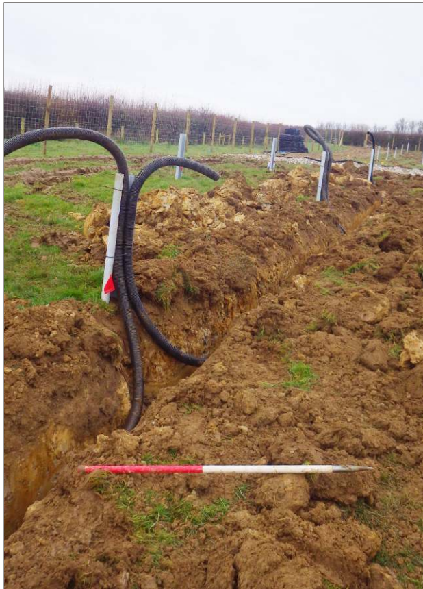
Plate 2: View of cable trench with ditch F103 visible in section. View to north-northwest (scale 1m)
