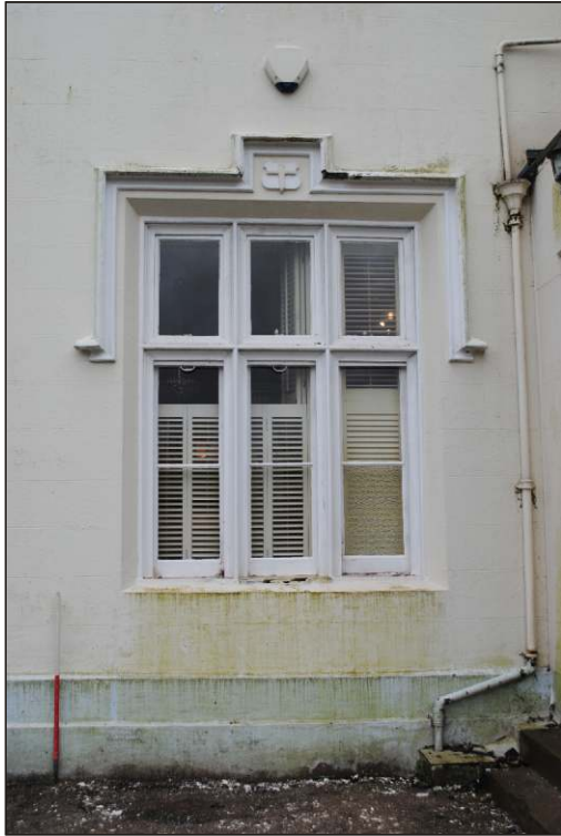
Plate 4: The ground floor window with a cross in shield design above and simple protruding stops to the drip mould with vertical cracks indicating the former larger opening, looking southeast. (1m scale)
