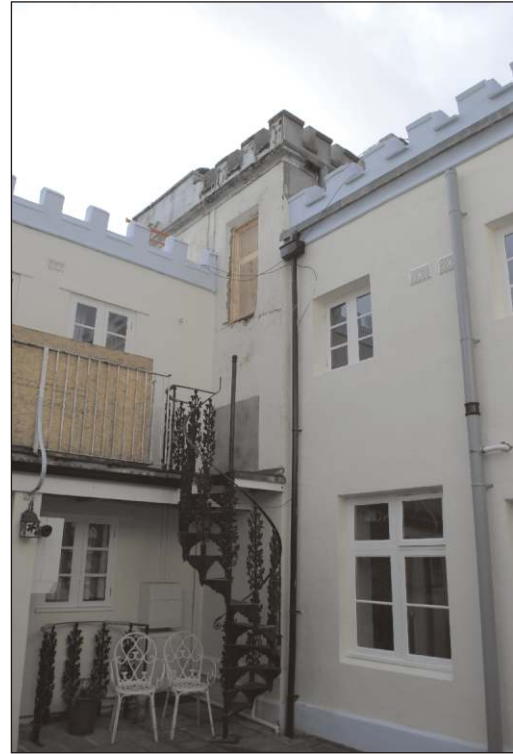
Plate 9: East courtyard wing showing primary work in southwest corner beyond the black drain pipe, looking southwest
