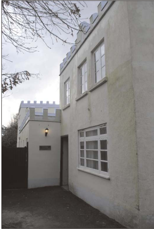
Plate 8: The northeast elevation of the east courtyard wing showing ground floor window in blocked arched opening and entrance to courtyard beyond, looking southwest. (1m scale)
