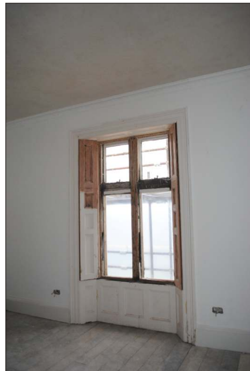
Plate 18: Shuttered and panelled walk in window in the south wall of the first floor southwest room (65/66)
