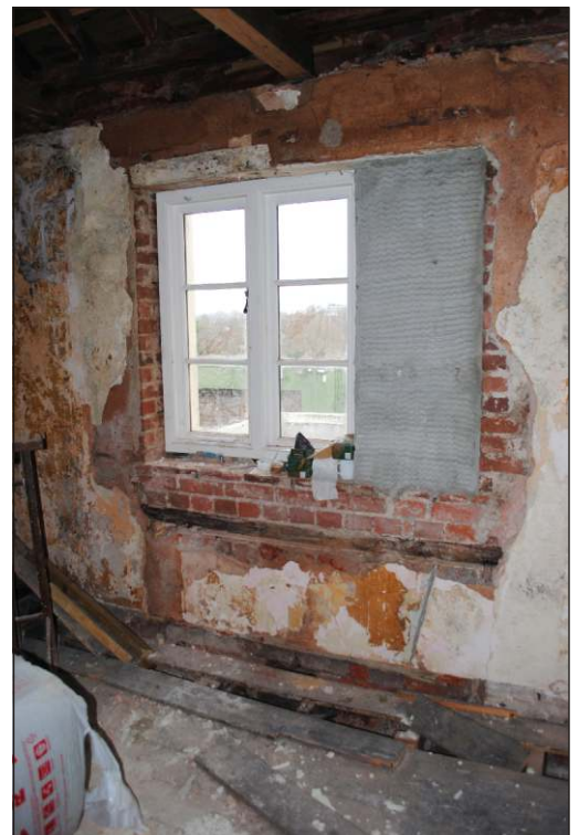
Plate 22: North wall of room (84) on first floor of the east courtyard wing west range, showing modern inserted window and blocked window below, looking northwest.
