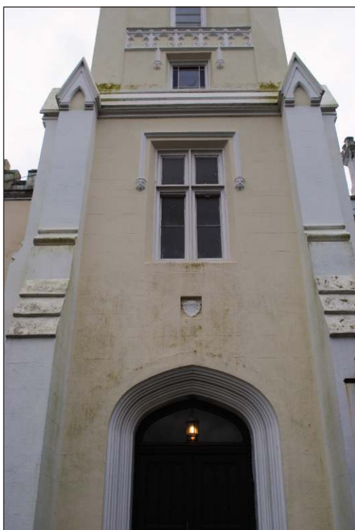
Plate 3: The northwest elevation showing the second-floor tower window and scallop shell in niche above the main entrance to the house
