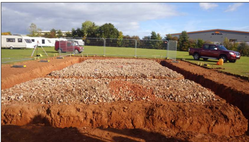
Plate 3: Showing footings trenches for reception building. View to east (scales 2 x 1m)
