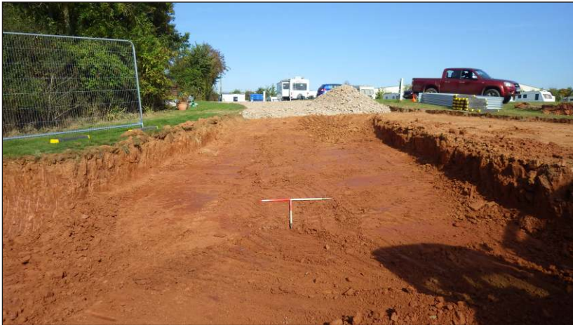
Plate 2: Showing ground reduction for storage building. View to northeast (scales 2 x 1m)
