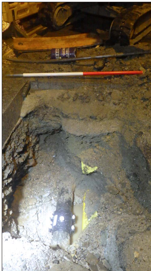
Plate 2. Showing monitored trench with water main exposed. View to south (scale 1m)
