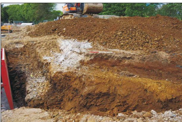
Plate 4: Excavation of the sewer trench along the northeast part of the site, looking northeast
