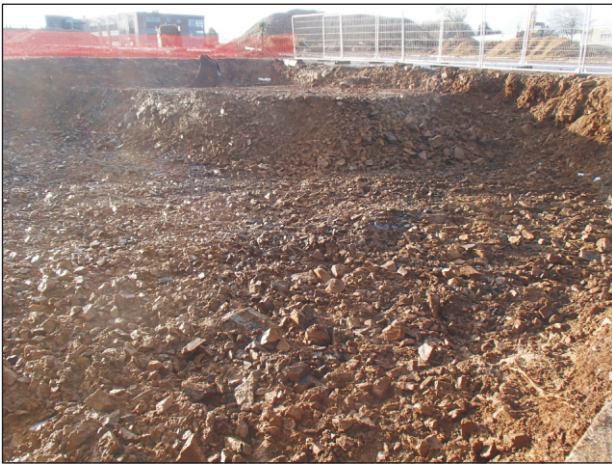
Plate 2: Disturbance adjacent to the northern access road, looking northwest
