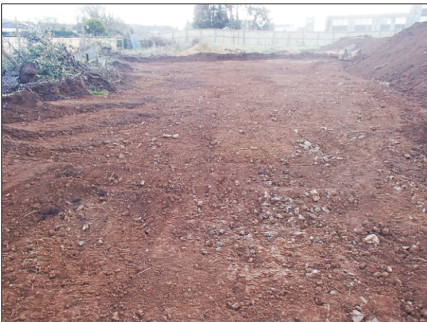
Plate 3: General view of topsoil stripping along the northeast part of the site, looking south
