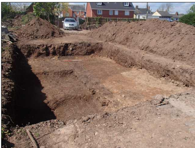
Plate 3: General view of excavation area in Trench 4, showing pit F405, looking northwest (scale 1m)
