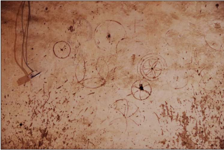
Plate 5: Detail of marks at west end of north elevation, looking north-northwest
