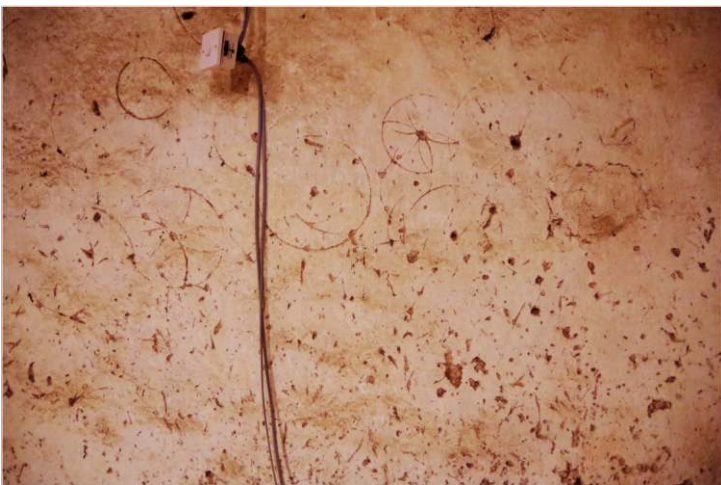
Plate 7: Detail of marks at east end of north elevation, looking north-northwest
