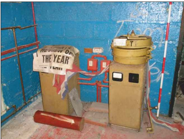
Plate 19: The two arc rectifiers in the southwest corner of the projector room, looking west-southwest. (1.4m scale)
