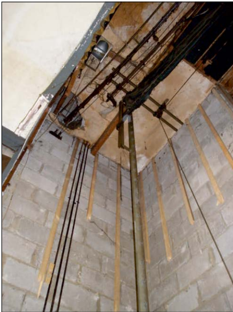
Plate 12: Detail of the fly space, north side of the stage, looking northeast
