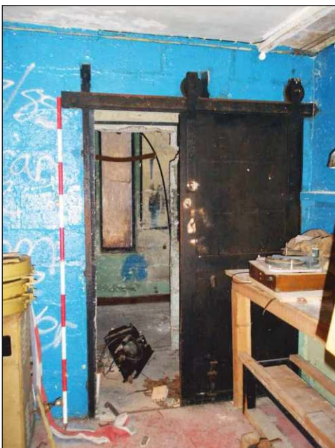
Plate 16: Detail of metal sliding doors at the north end of the west elevation of the projector room, looking west. (2m scale)
