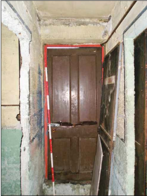
Plate 14: First-floor corridor, view of door to roof terrace, looking north-northwest. (2m scale)
