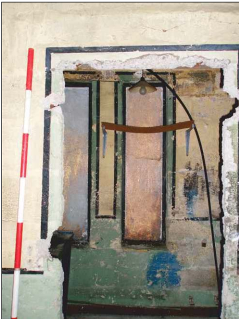
Plate 15: View from the first-floor corridor of windows in west elevation and original Art Deco style wall paint, looking west-southwest. (1.2m scale)
