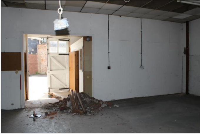
Plate 29: Unit 6, view to offices along southwest interior elevation, looking southwest. 1m scale
