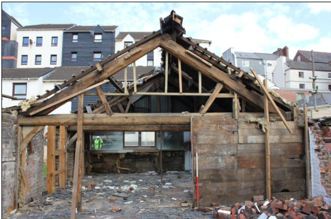
Plate 24: Unit 2 looking to Unit 3, second floor, detail of original A-frame truss, looking northeast. 1m scale
