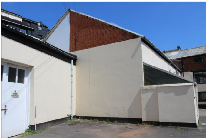
Plate 7: Northwest exterior elevation of Unit 5 and the southwest elevation of Unit 6, looking east. 1m scale
