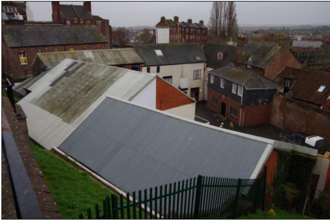
Plate 9: Northeast exterior elevation of the north range obscured by topography, with general view to Eagle Yard, looking south
