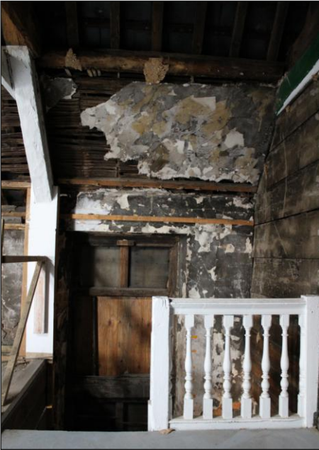
Plate 22: Unit 1, second floor, southeast elevation at southwest end showing lath and plaster, looking southeast
