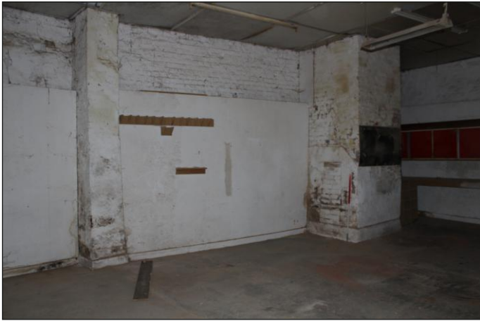
Plate 25: Unit 3, ground floor, brick furnace against the southeast elevation, looking south. 1m scale
