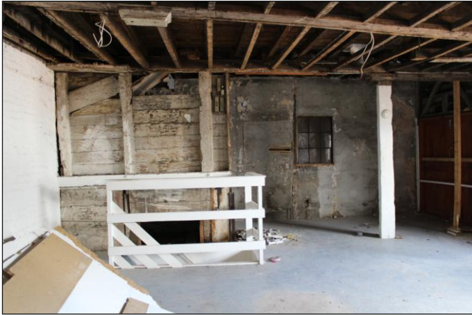
Plate 18: Unit 1, first floor, southwest elevation showing mid-18th-century wall and mid to late 18th-century timber panelling of staircase, looking southwest
