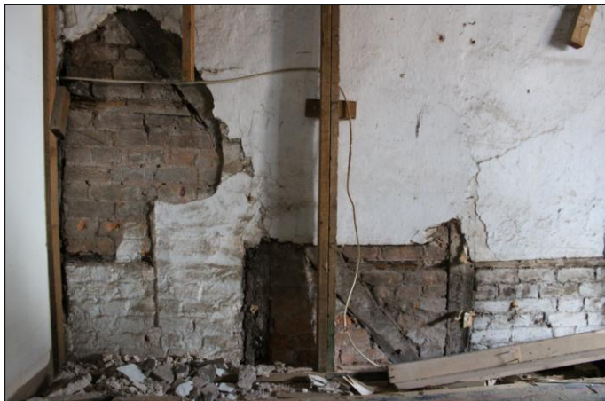
Plate 16: Unit 1, ground floor, southwest elevation showing mid 18th-century timber and brick wall with plaster finish, looking southwest
