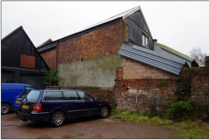
Plate 5: Southeast exterior elevation of the south range at the northeast end, looking west-southwest. 1m scale
