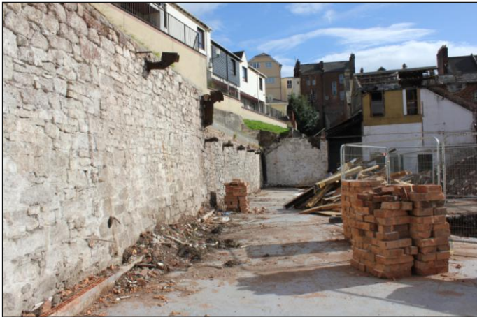
Plate 10: View along northeast breccia boundary wall, with in situ corbel-like iron braces of the mid-19th-century foundry, looking east
