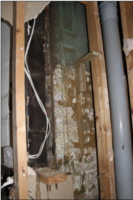
Plate 13: Unit 1A, timber panelling in the south corner of the ground floor, looking east-southeast
