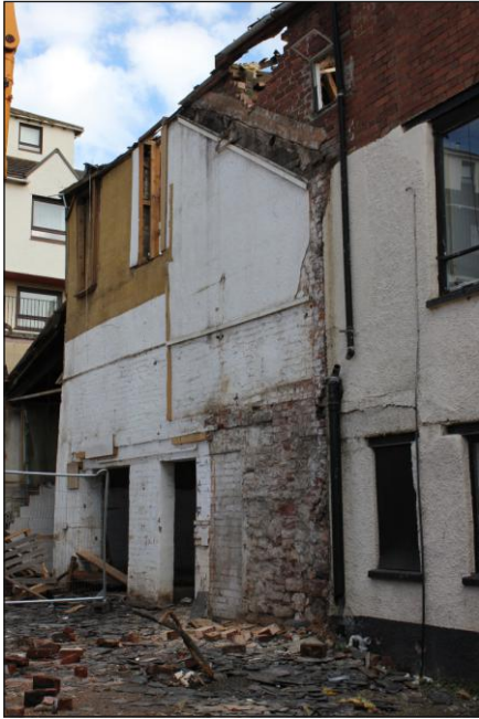
Plate 26: Unit 3, during demolition, showing breccia masonry incorporated into the early 19th-century wall of the south range, looking east
