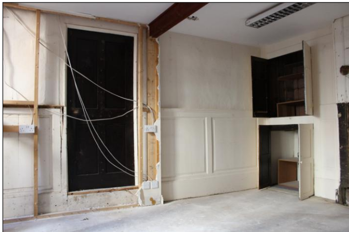
Plate 14: Unit 1A, northeast elevation showing timber panelling and doorway to Unit 1, looking east
