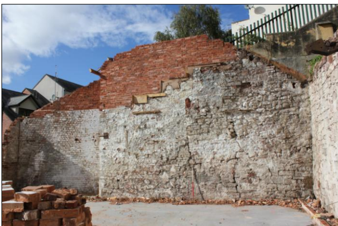
Plate 8: Northwest elevation of mid-19th-century foundry building taken during demolition, showing the earlier boundary wall, looking
