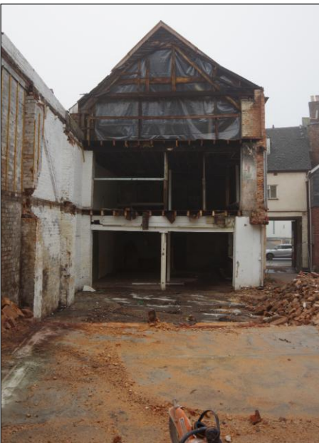
Plate 3: Northeast gable end of the early 19th-century section of the south range showing the original truss and alterations to the northwest side, looking northeast
