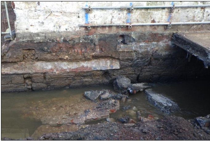
Plate 37: Higher Leat, transition from Zones 5 to 6 showing where line for brick vaulting ends, looking northeast
