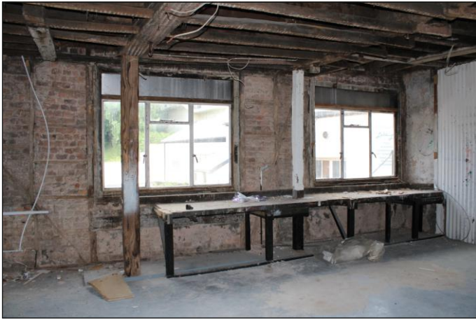
Plate 17: Unit 1, first floor, northwest elevation, showing mid to late 18th-century timber and brick wall, looking north
