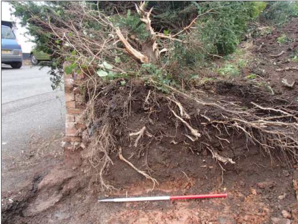
Plate 2: Section through breached brick wall. View to south (Scale 1m)
