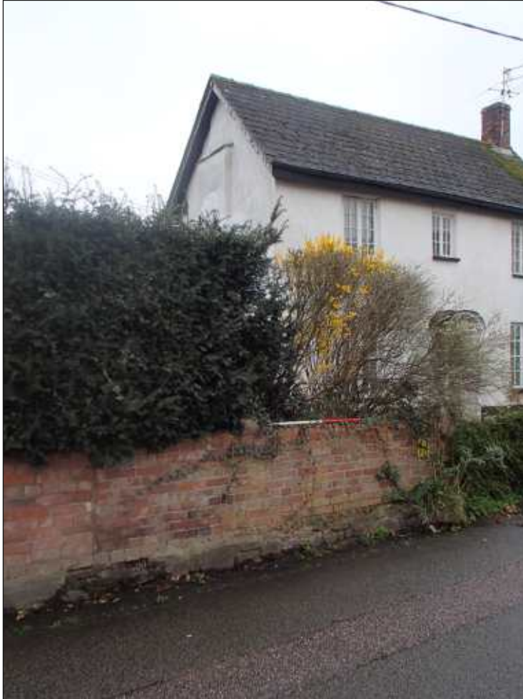
Plate 1: Showing Howden Lodge with pre-excitation view of brick wall breach position. Looking northwest (Scale 1m)
