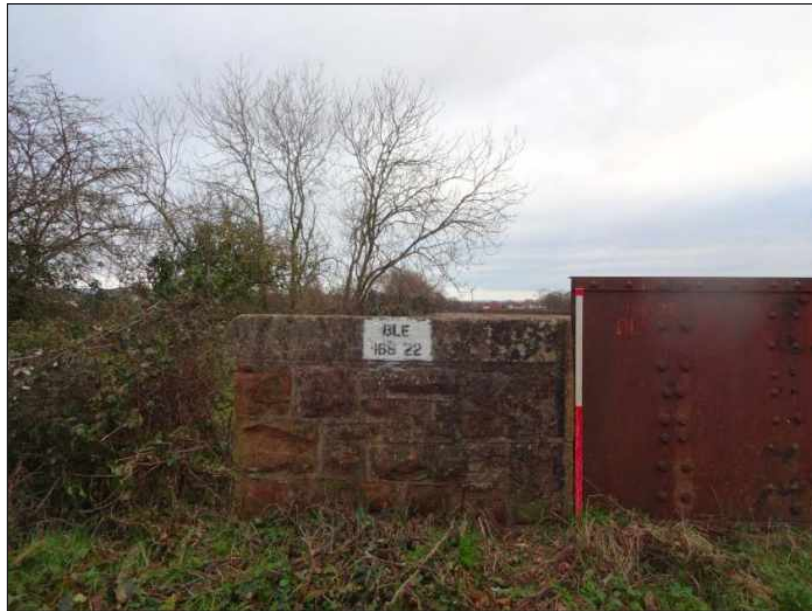
Plate 7: North end of parapet showing the bridge number, viewed from the west (scale 1m)
