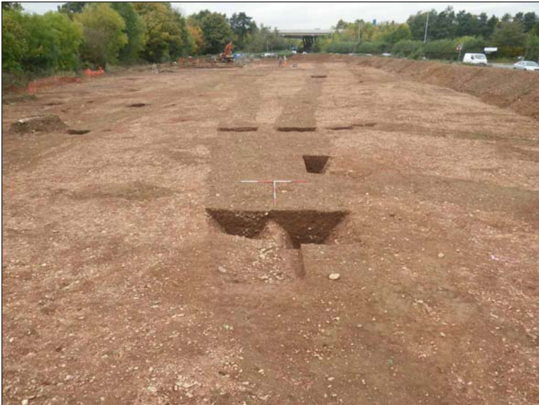
Plate 4: General view of ditches F107 and F108, looking northwest (2 x 2m scales)
