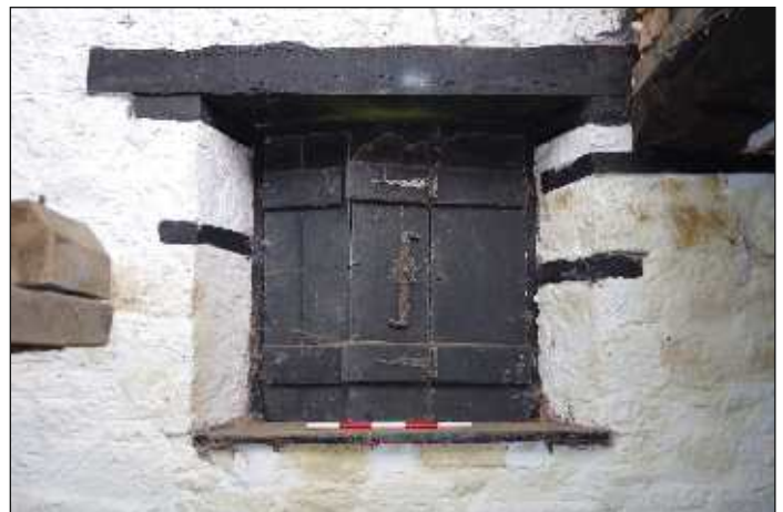
Plate 16: Window on the northeast elevation of the cider press room, with detail of the timber shutters, looking northeast. 0.5m scale
