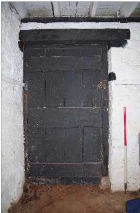
Plate 15: Plank and batten door, leading to the barrel/cask store room, looking northwest. 1m scale
