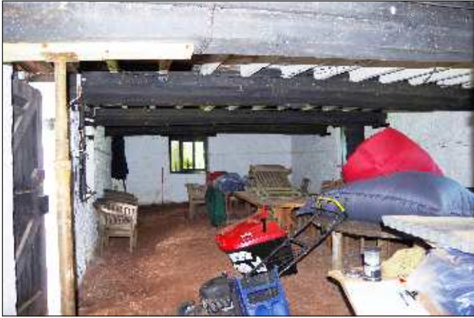
Plate 21: General view to the northwest end of the barrel/cask store room, looking northwest. 1m scale
