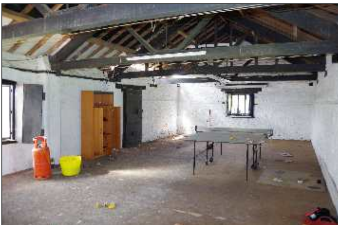
Plate 24: General view to the northwest end of the northwest room of the first floor, looking west. 1m scale
