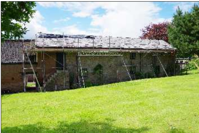
Plate 6: Northeast elevation of the cider barn and the cob wall of the stable block within the linhay, looking southwest. 1m scale
