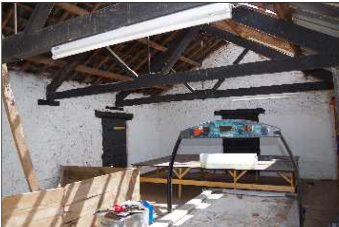
Plate 27: General view to the southeast end of the first-floor southeast room, looking east
