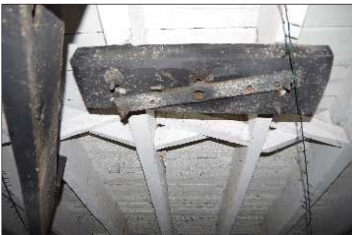
Plate 20: Fixtures on the ceiling to the south of the cider press, associated with the ratchet mechanism of the press, looking northwest
