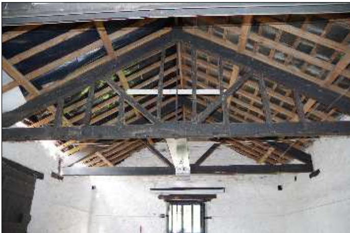
Plate 26: Detail of the truss with evidence for a former partition located towards the northwest end of the first-floor northwest room, looking northwest
