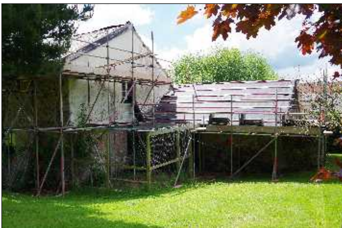
Plate 8: Northwest elevation of the cider barn and the chicken coop extension, looking south-southeast
