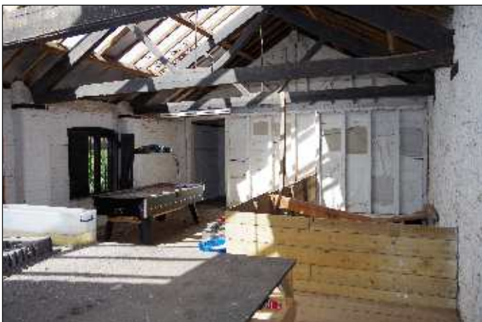
Plate 28: General view to the northwest end of the first-floor southeast room, looking northwest
