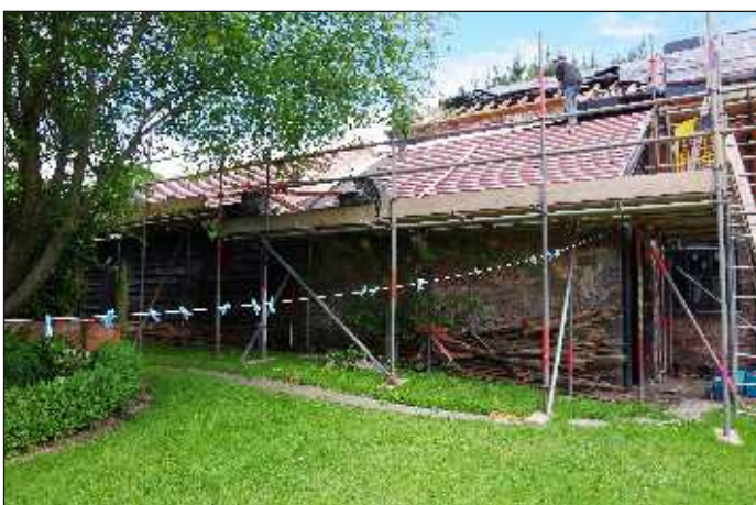
Plate 4: Northwest end of the southwest elevation, showing extensions, looking north. 1m scale
