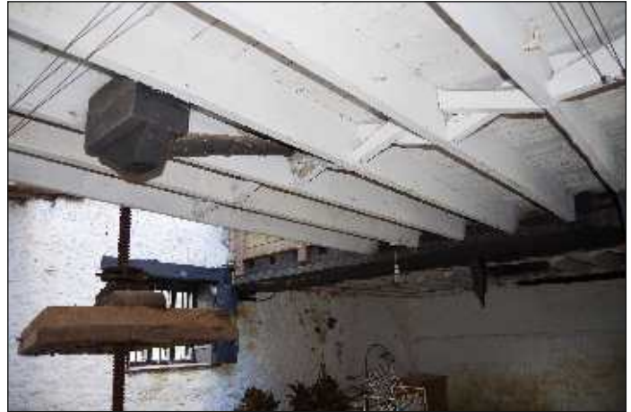
Plate 18: Fixtures on the ceiling to the southwest of the cider press, associated with the ratchet mechanism of the cider press, looking northeast
