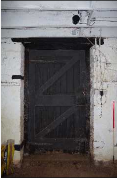
Plate 13: Plank and batten door with ledges and braces, leading to the exterior from the cider press room, looking southwest. 1m scale
