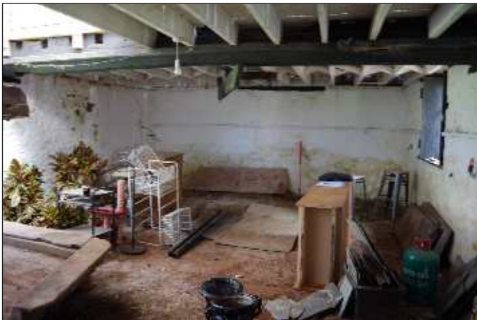
Plate 11: General view to the southeast end of the cider press room, looking east. 1m scale
