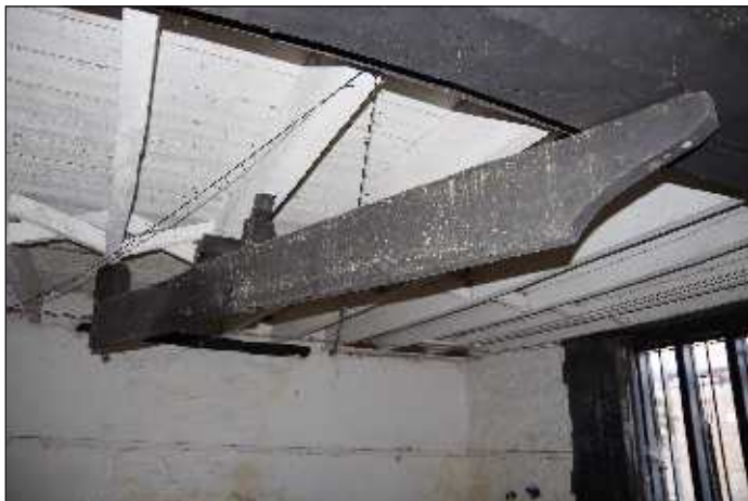
Plate 19: Fixtures on the ceiling to the south of the cider press, associated with the ratchet mechanism of the press, looking south
