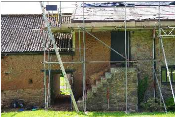
Plate 7: Close-up of the southeast end of the northeast elevation of the cider barn, showing the cob abutted by the Raddon stonework, looking southwest. 1m scale
