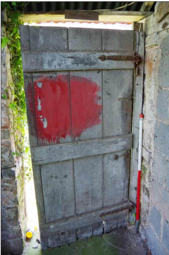
Plate 28: Detail of plank and batten door on east elevation of the outbuilding, looking east-southeast. (1m scale)
