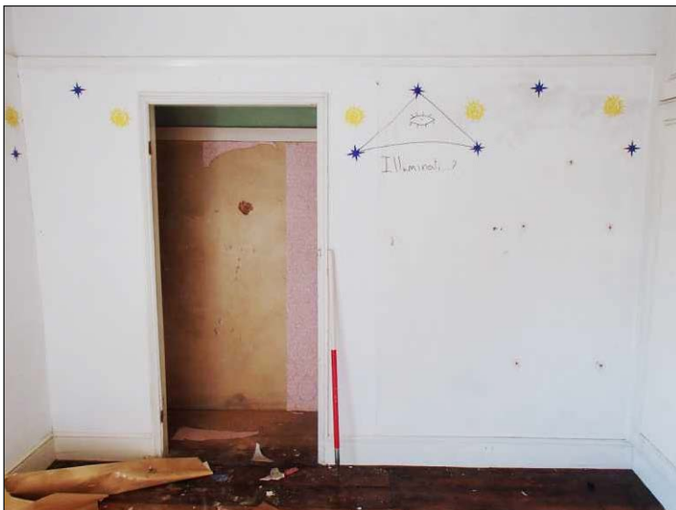
Plate 19: Room 7, showing recess at east end of south elevation and blocked fireplace to west side, looking south-southwest. (1m scale)
