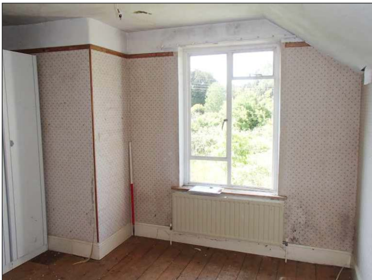
Plate 20: Room 8, showing blocked fireplace at east end of the south elevation, looking south. (1m scale)
