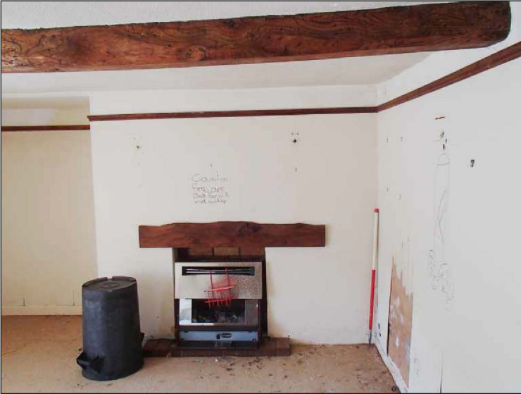
Plate 13: Room 2, showing earlier chimney breast along the south elevation and the chamfered beam, looking south-southwest. (1m scale)
