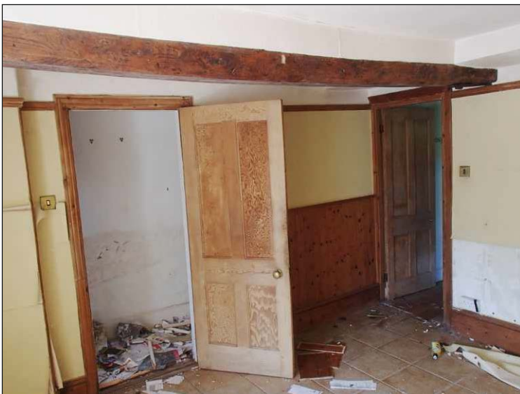
Plate 11: Room 1, showing chamfered beam, stripped timber doors, wainscoting, skirting and picture rail, looking southwest
