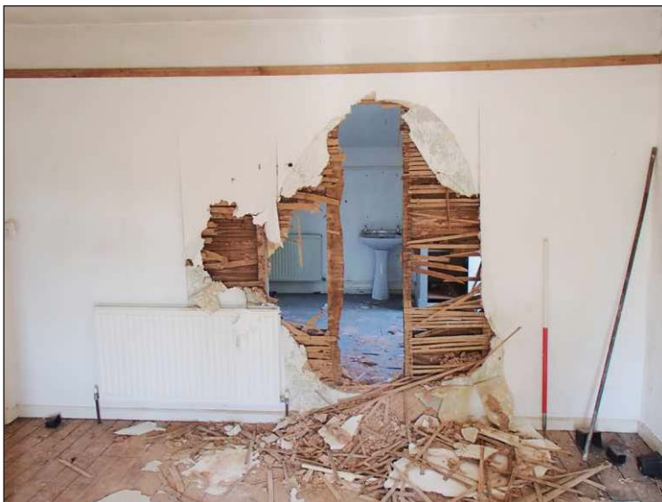
Plate 17: Room 5, showing the lath and plaster west partition wall, looking west-northwest. (1m scale)
