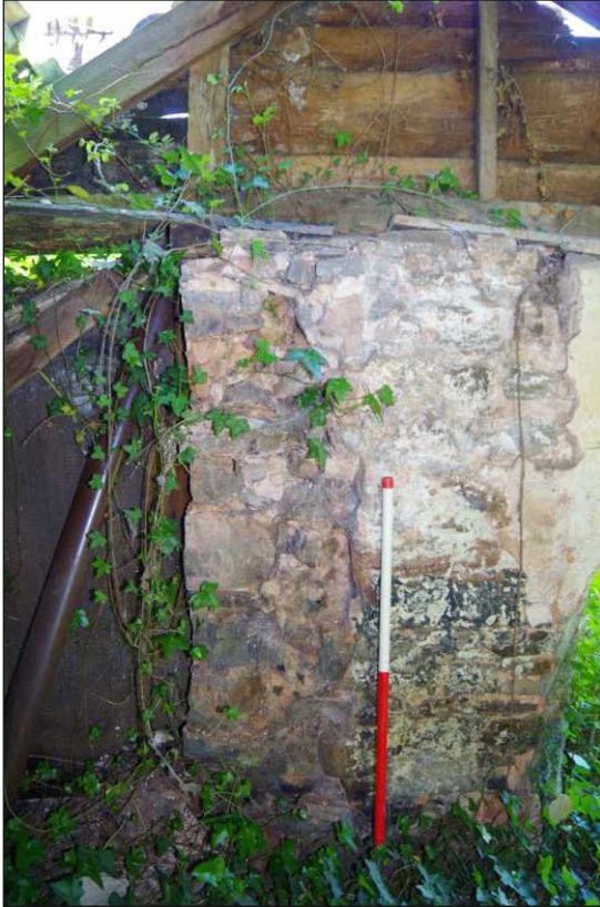
Plate 27: Internal stub wall towards west end of the north elevation, north-northeast. (1m scale)
