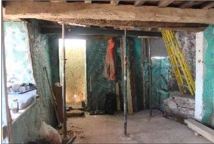
Plate 3: The ground floor showing the inserted openings in the south elevation, looking south. 1m scale
