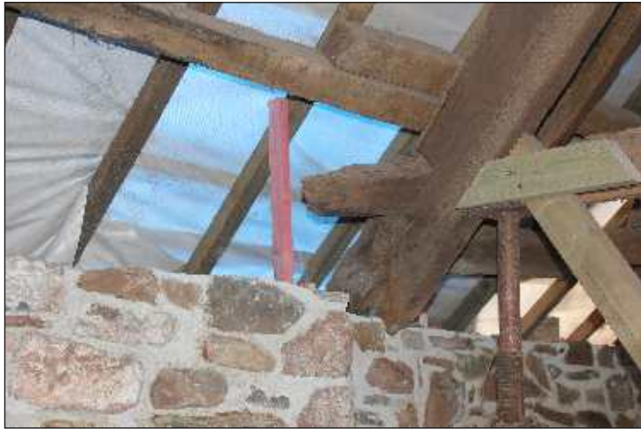
Plate 14: Close-up of the roof details in the bay over the chimney stack, looking northwest
