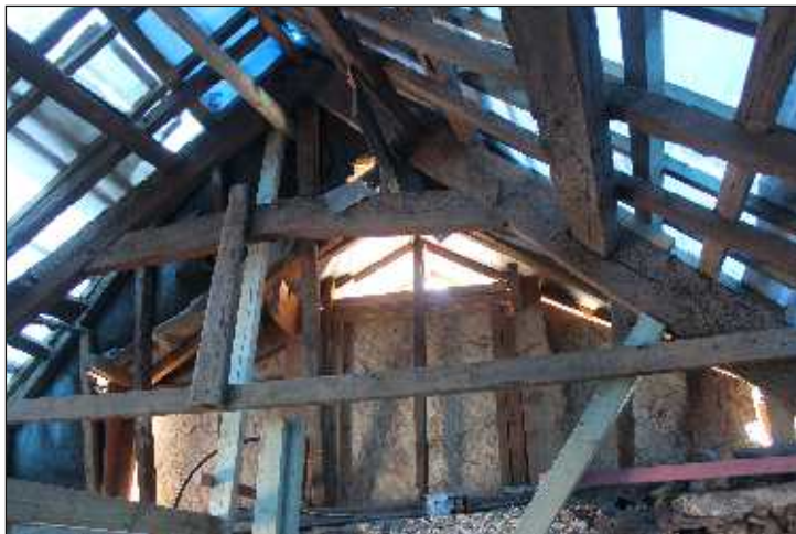
Plate 13: The south truss, showing cambered collar, lapped apexes and the through purlins, looking south
