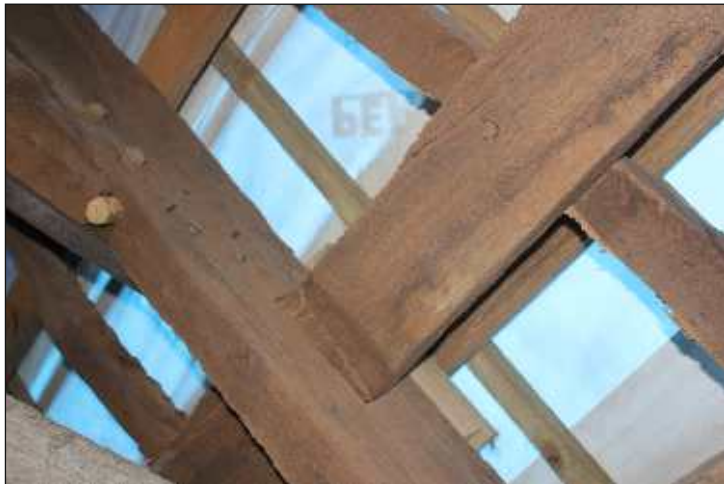
Plate 15: Close-up view of the roof showing collar joint, lapped purlins and pegged secondary rafter, looking northeast
