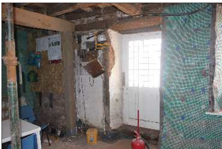
Plate 4: The ground-floor east wall showing narrower masonry adjacent to the front door, looking northeast. 1m scale
