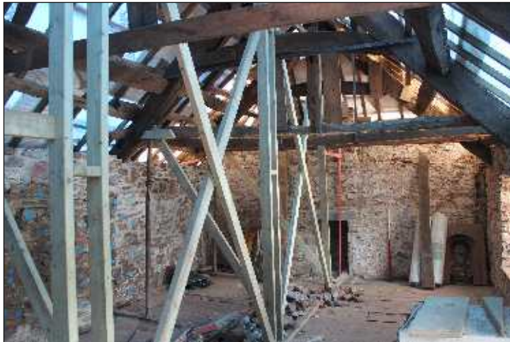
Plate 9: General view of the first floor showing stack to left and fireplace in the north wall (centre) with removed grate to the right, looking north. 1m scale
