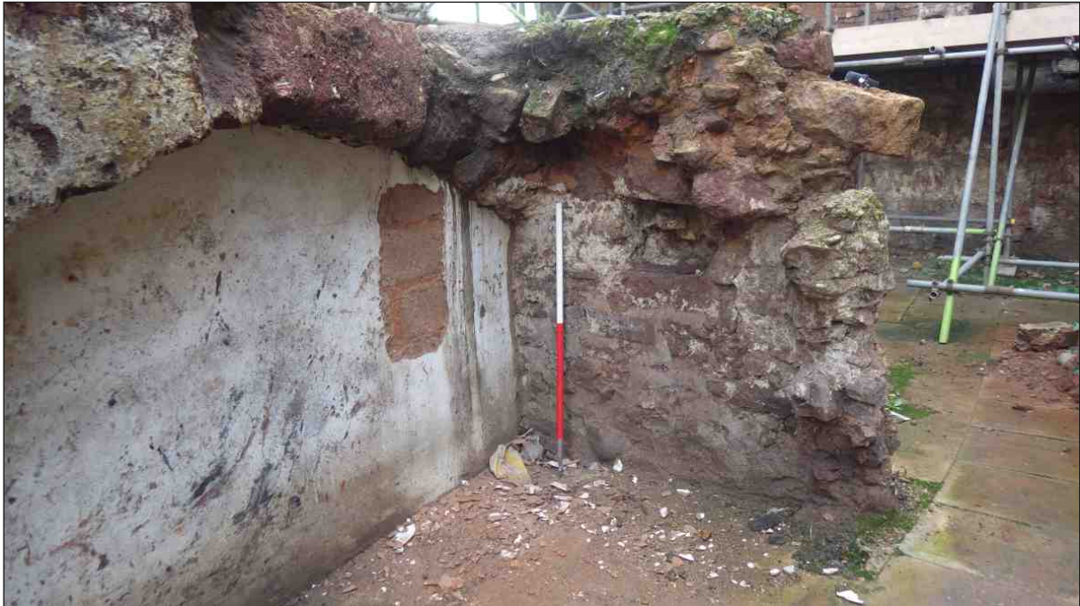
Appendix Plate 3: The east wall of the rear west cellar looking southeast showing the exposed concrete blocks. 1m scale
