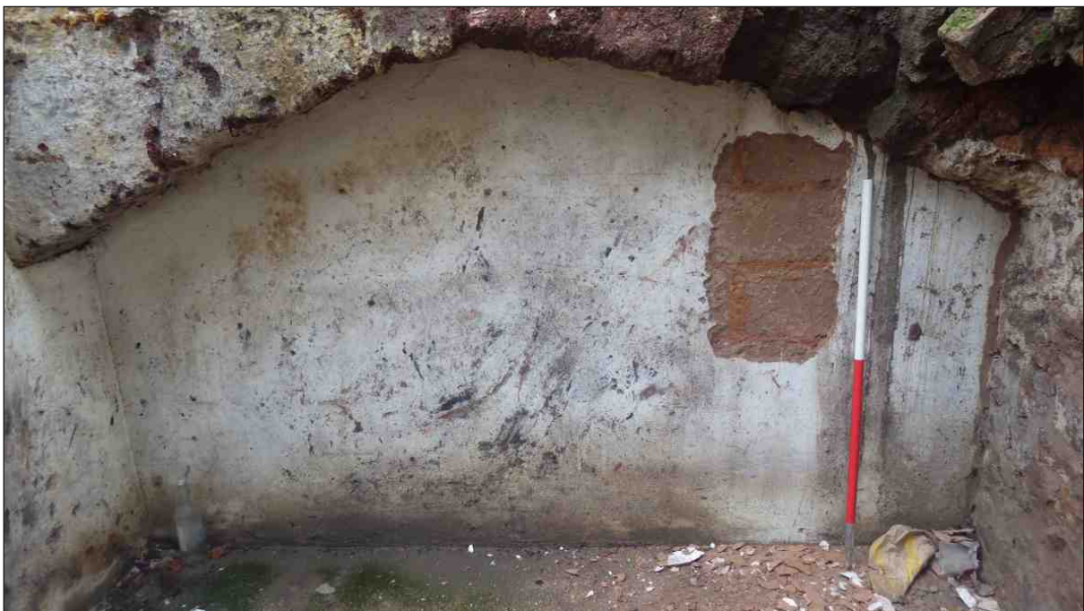
Appendix Plate 2: The east wall of the rear west cellar looking northeast showing the exposed concrete blocks. 1m scale
