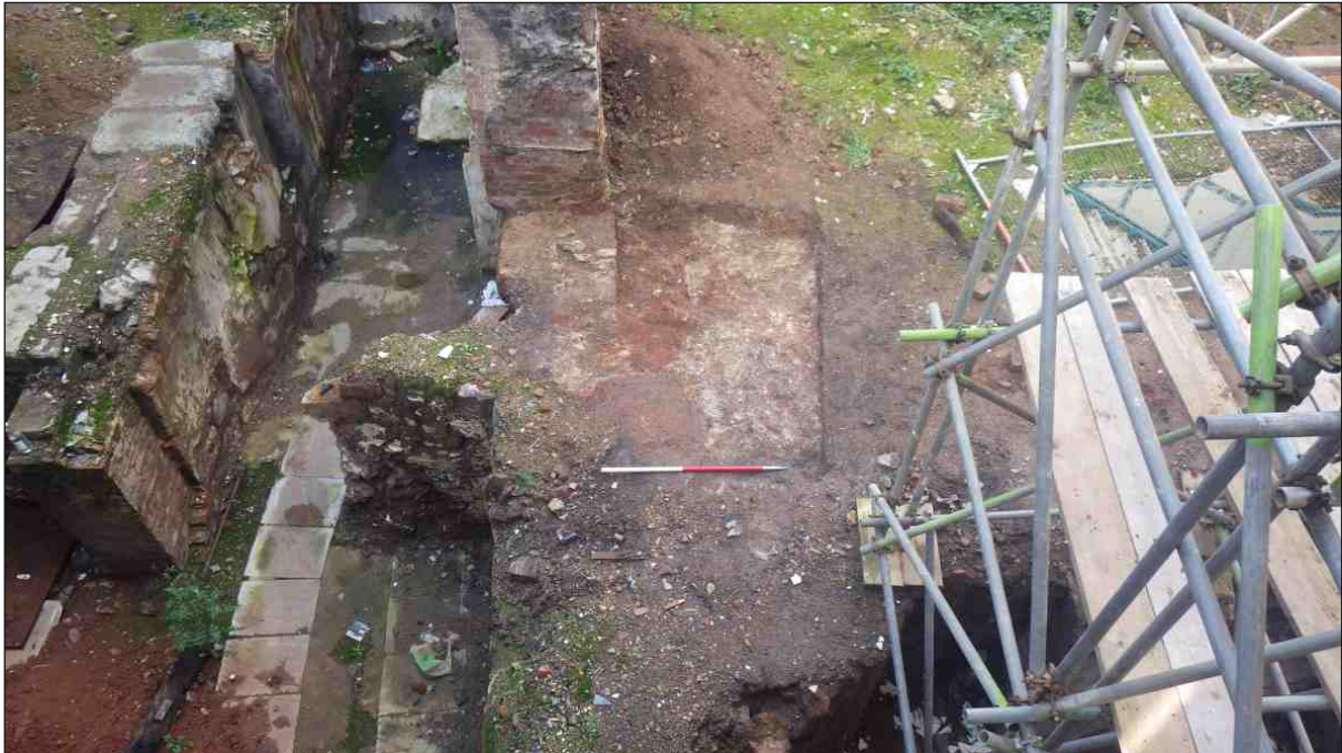
Appendix Plate 1: The investigations looking northwest down from the scaffolding showing wall 1307 below the scale, with wall 1306 above. 1m scale
