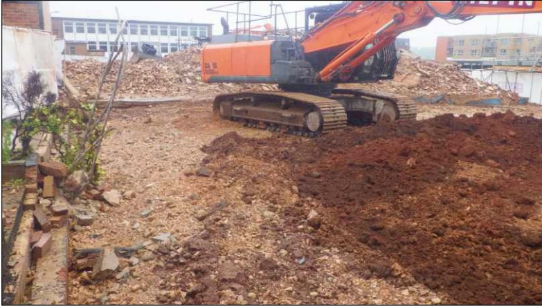
Plate 1: Watching brief area, southwest extent of the site, work in progress, looking northeast
