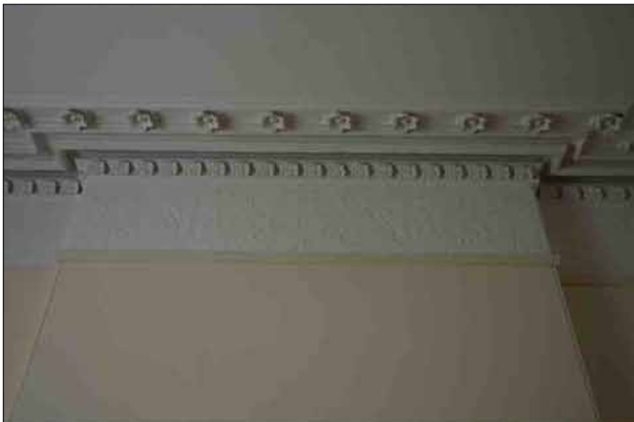
Plate 14: Decorative coving and embossed wallpaper in the western rooms on the ground floor, looking northwest
