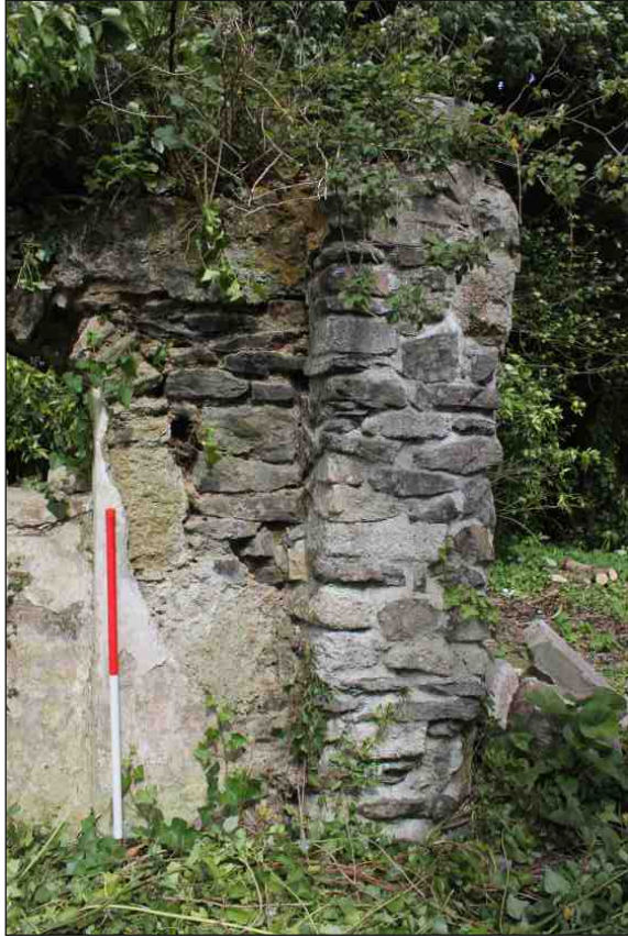
Plate 1: The west elevation of the boundary wall showing the rebuilt pier, looking east. 1m scale
