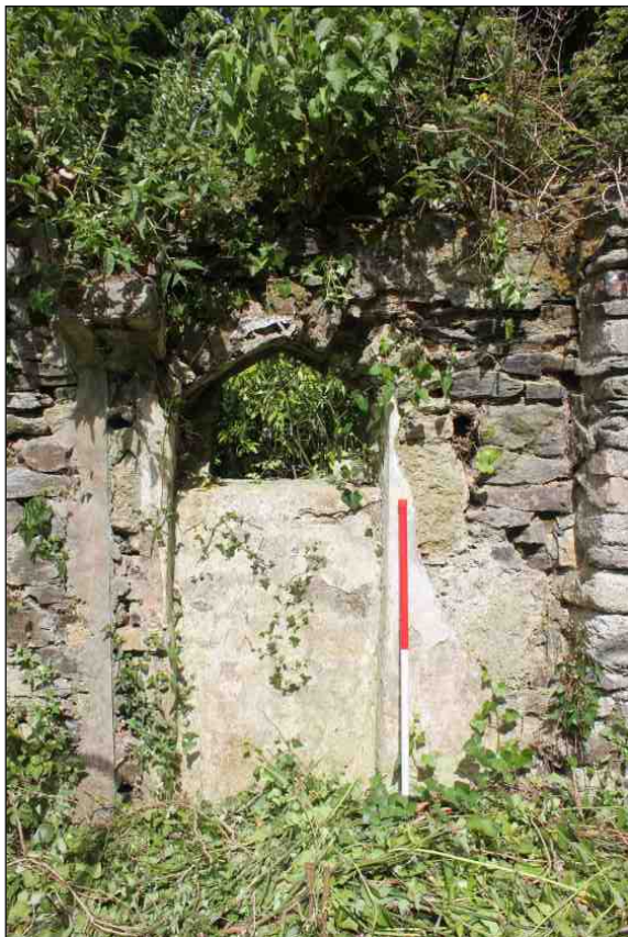
Plate 2: The west elevation of the boundary wall showing the blocked doorway, looking east. 1m scale
