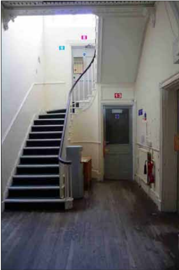
Plate 10: General view of stairs to the first floor, looking northwest (1m scale)
