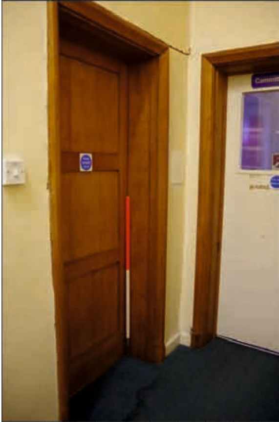
Plate 53: Original 3-panel door and surround on ground floor of the dining hall building, looking southwest (1m scale)
