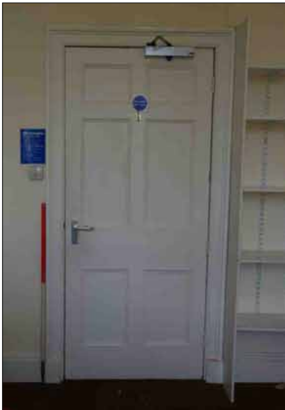
Plate 21: 6-panel door in surround on the first floor, looking northeast (1m scale)
