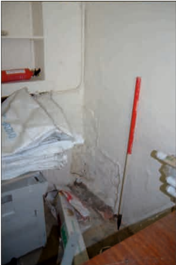
Plate 42: Scar of removed copper in the southeast room on the ground floor of the infill building, looking northwest (1m scale)
