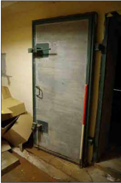
Plate 4: Blast door in the northeast room of the basement, looking northeast (1m scale)
