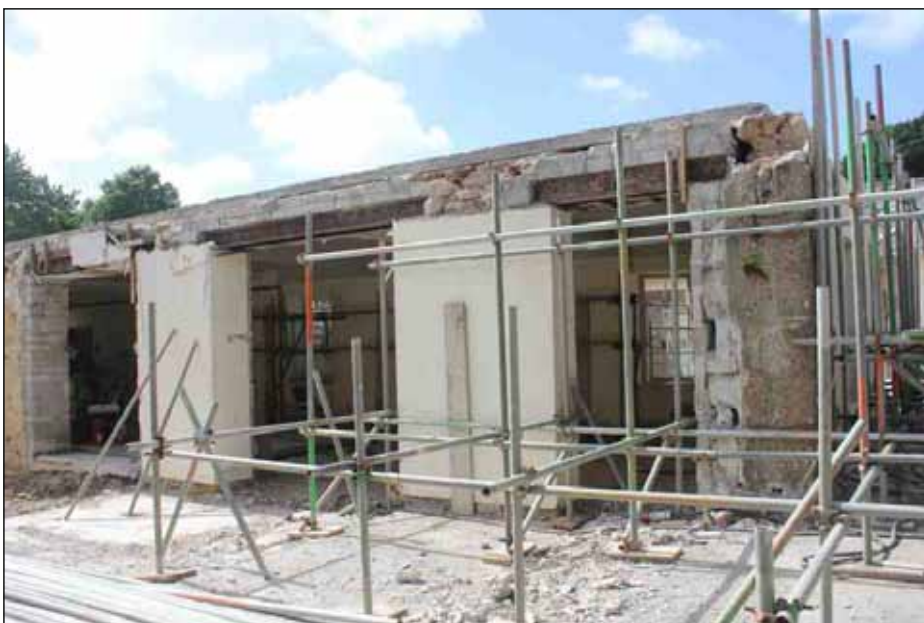
Plate 39: The south elevation of the original stable block following removed of the attached infill building showing modern openings, looking northwest
