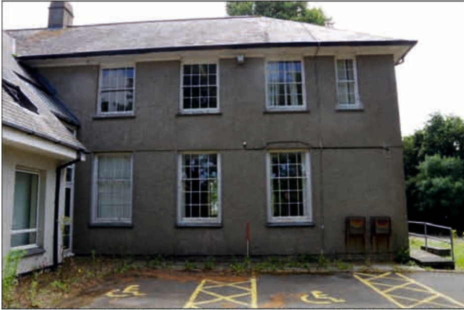
Plate 59: Southern end of the northwest elevation of the dormitory building, looking southeast (1m scale)
