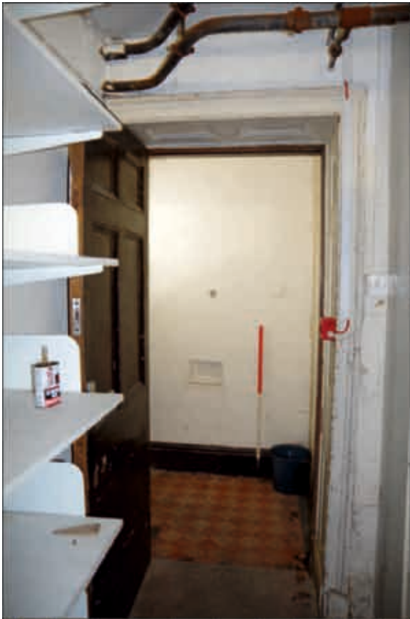
Plate 40: Lobby in the southwest room on the ground floor of the infill building, looking southwest (1m scale)
