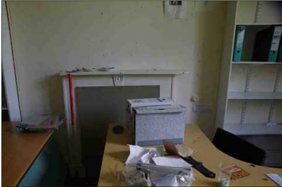
Plate 25: Fireplace in the northeast room on the first floor, looking northeast (1m scale)
