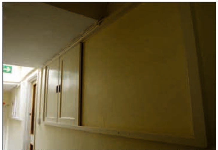
Plate 43: Two former serving hatches in the corridor on the first floor of the infill building, looking east
