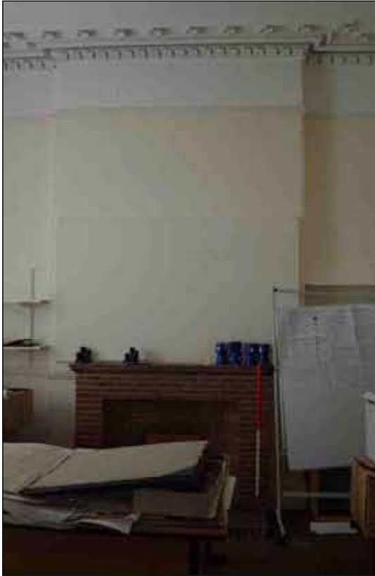
Plate 16: Fireplace in the northwest room on the ground floor, looking northwest (1m scale)
