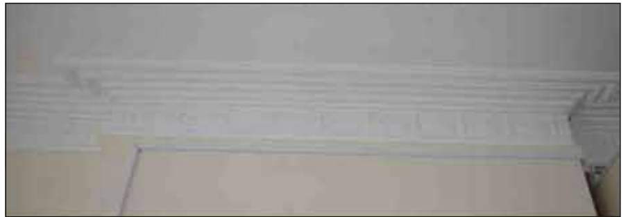
Plate 20: Ceiling border and embossed wall paper seen in the western rooms on the first floor, looking northwest
