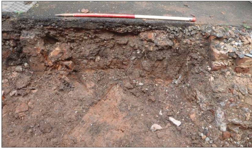
Plate 7: Representative section of foundation trench in block J, looking northwest (1m scale)
