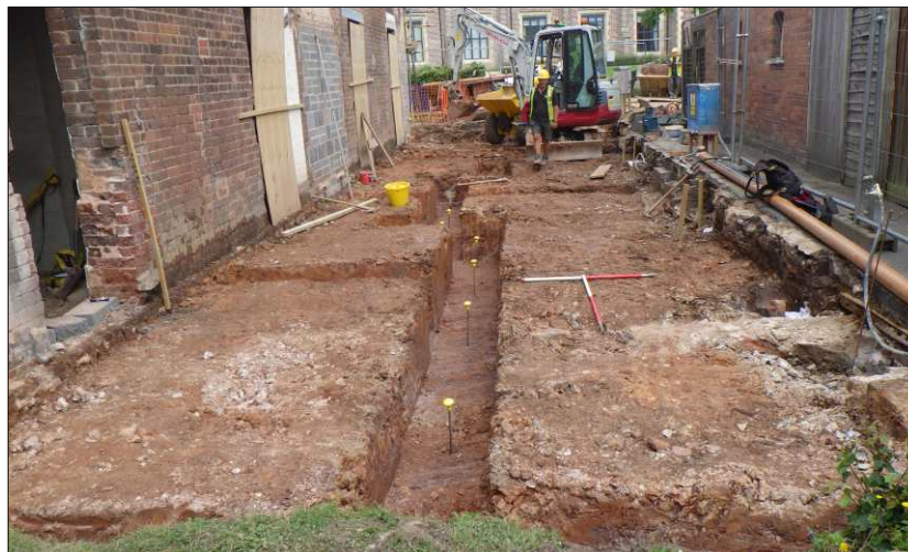
Plate 12: Working shot of foundation trenches being excavated in block A, looking northeast
