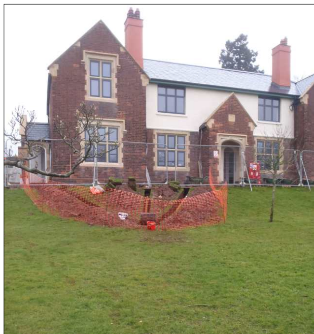
Plate 3: General view of drainage trenches situated to the southwest of block H, looking northwest
