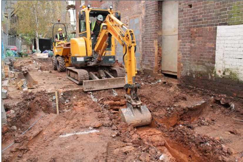
Plate 1: Working shot of foundation trenches being excavated in block H, looking east
