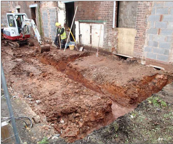
Plate 10: Working shot of foundation trenches being excavated in block F, looking southwest
