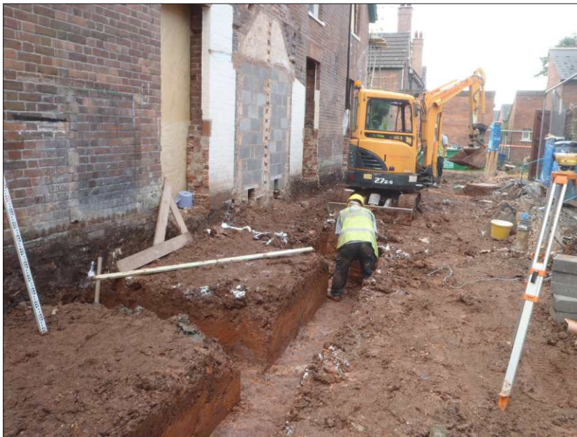
Plate 6: Working shot of foundation trenches being excavated in block J, looking southwest
