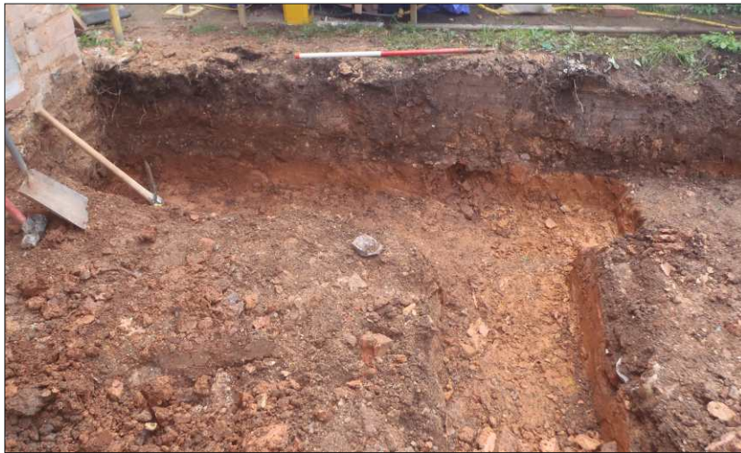
Plate 2: Representative section of foundation trench in block H, looking southwest (1m scale)
