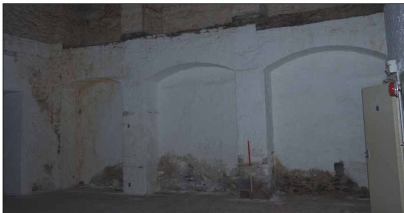
Plate 6: Ground-floor east wall in the south store on the ground floor, looking northeast (1m scale)
