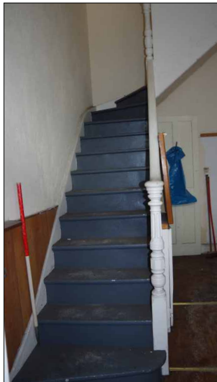
Plate 5: Stairs in the office on the ground floor, looking north (1m scale)
