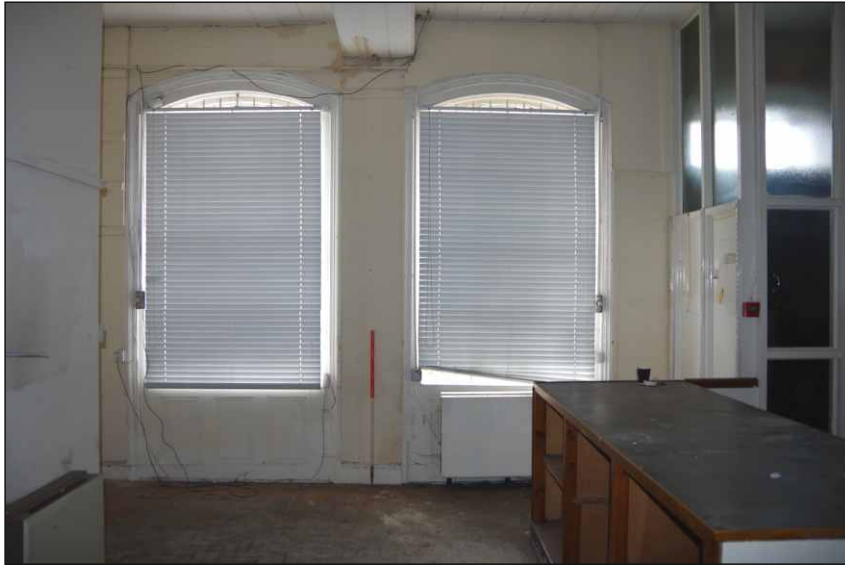
Plate 4: South wall of the office on the ground floor, looking south (1m scale)
