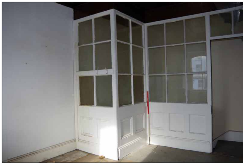
Plate 11: Partition in southwest office on the first floor, looking northwest (1m scale)
