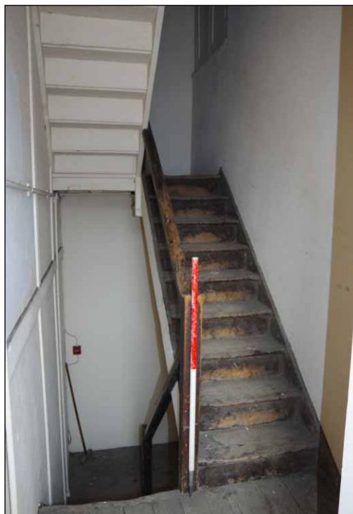
Plate 12: General view of stairs in the southeast corner of the building, looking north (1m scale)
