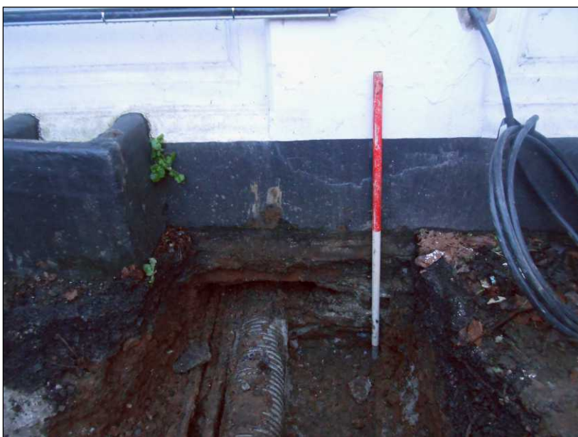
Plate 5: The existing cable where it enters 4 Abbey Place, looking southeast. 1m scale
