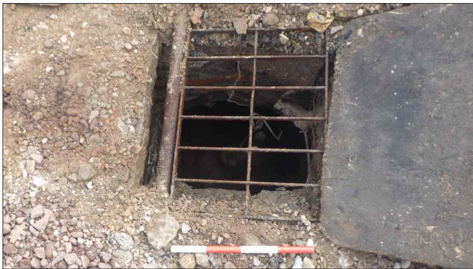
Plate 7: Manhole for access to subterranean tank, looking southeast (0.4m scale)
