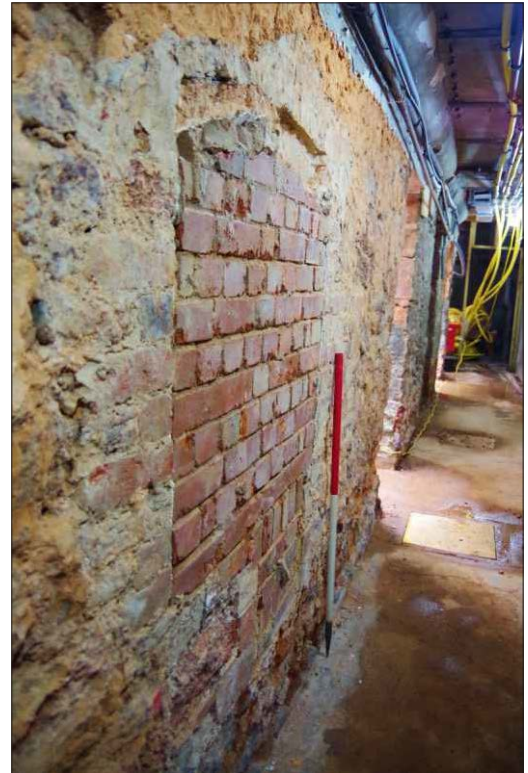
Plate 18: Basement passage under Lamb Alley showing infill behind the fireplace, looking west. (1m scale)
