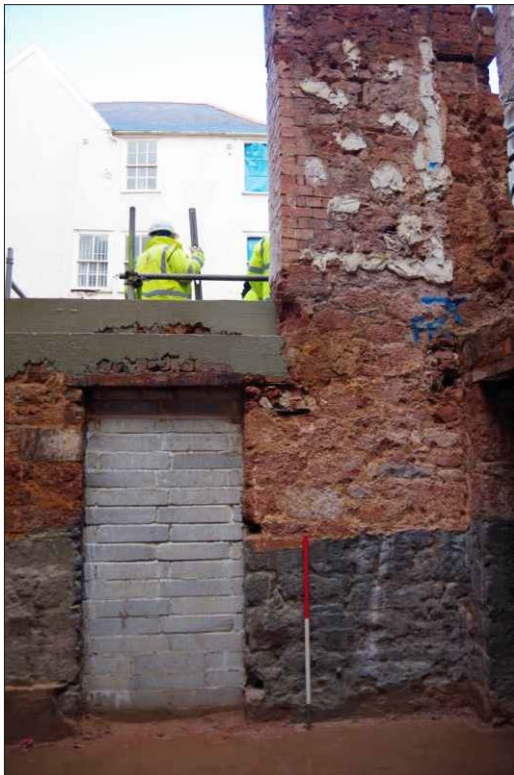
Plate 11: The middle basement, east end of the northwest wall, looking northwest. 1m scale
