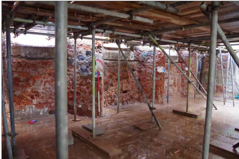
Plate 2: The rear basement, northeast wall showing former cellar lights, looking east. (1m scale)
