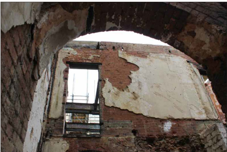
Plate 35: The ground floor, north range, east side of southeast wall, looking northwest
