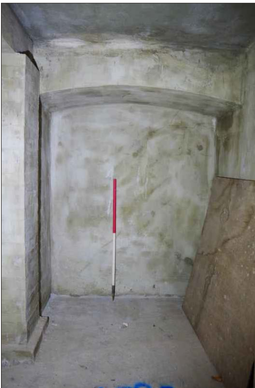
Plate 20: A typical arched recess in the front wall under the front yard, looking southeast. (1m scale)
