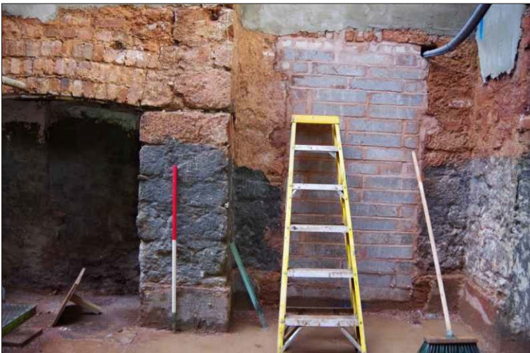
Plate 15: The front basement, blocked doorway in the northeast wall, looking northeast. (1m scale)
