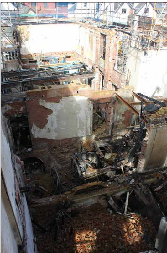
Plate 22: Pre-clearance view through the building looking down from the second floor to the ground-floor front range, looking north-northeast
