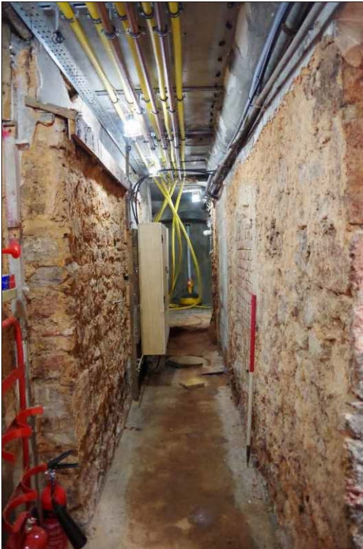
Plate 17: Basement passage under Lamb Alley showing break in northeast wall, looking southeast. (1m scale)
