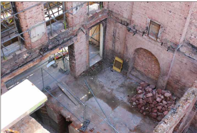
Plate 23: The ground-floor front range following clearance showing the brick southwest elevation, and the stone southeast elevation, looking south
