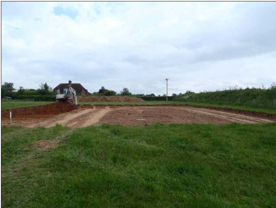
Plate 1: General view of area stripped for new dwelling. Looking northwest (scales 2 x 1m)
