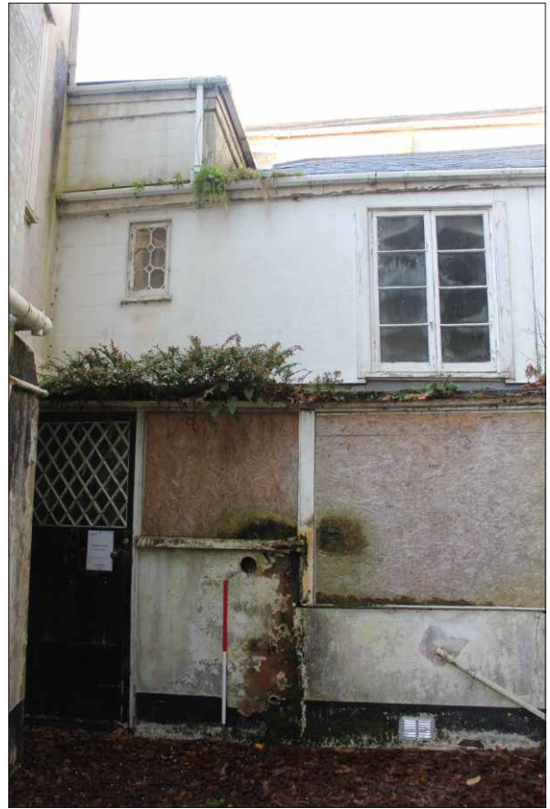
Plate 14: The east elevation of the rear service range, looking west (1m scale)
