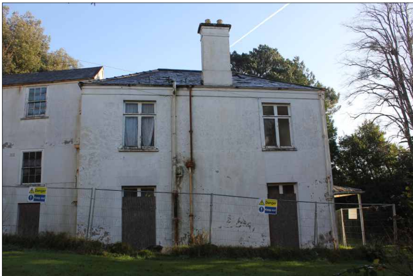
Plate 6: The west elevation of the front range of the house, looking east
