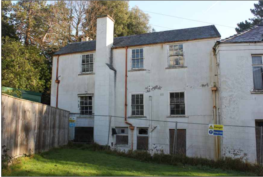
Plate 7: The west elevation of the rear service range of the house, looking east
